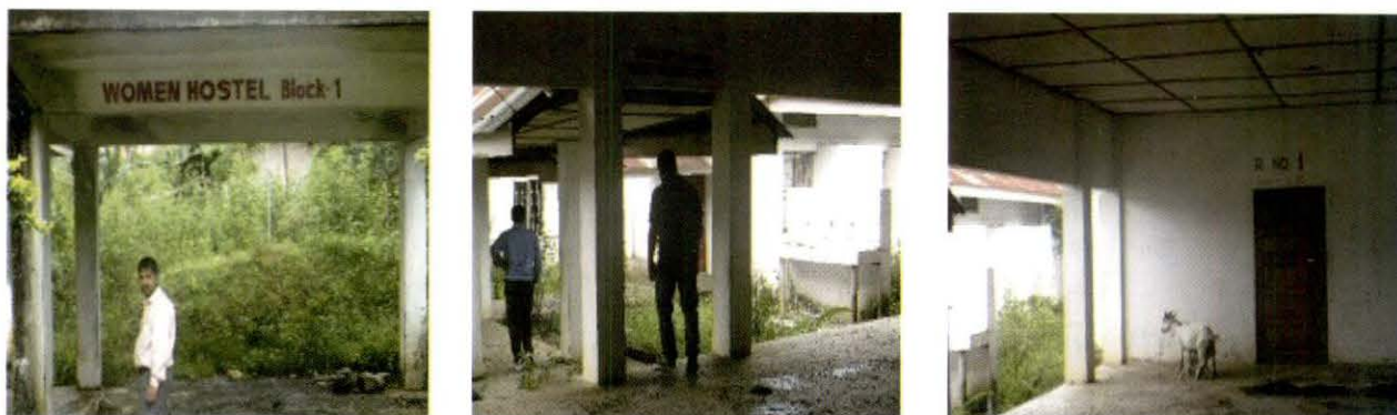
Poor maintenance of Women hostel at Yupia
