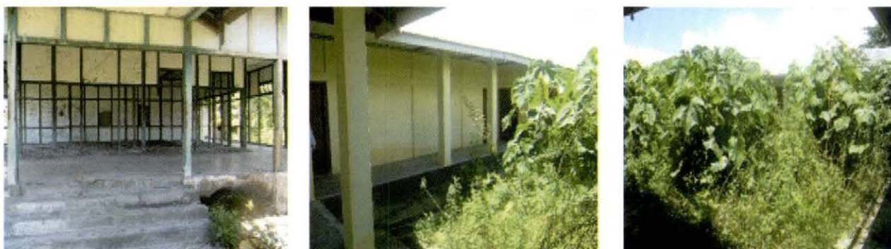
Dilapidated old Hostel Building and New Hostel Building indicating lack of maintenance.
