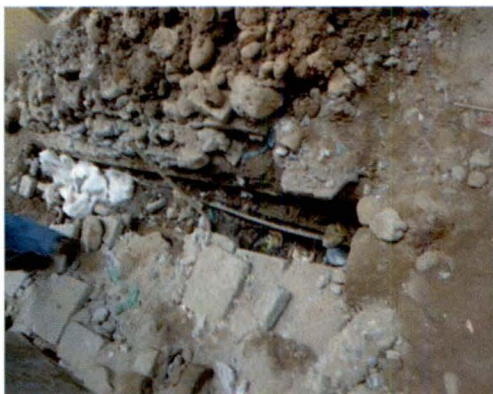
Work held up due to non-shifting of underground utilities by PHE, BSNL. (Jammu & Kashmir)
