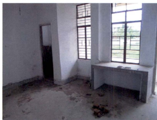
Nagaland- BSUP project, Kohima: DU constructed with single room at Burma Camp- Photo Taken on 08/06/2011
