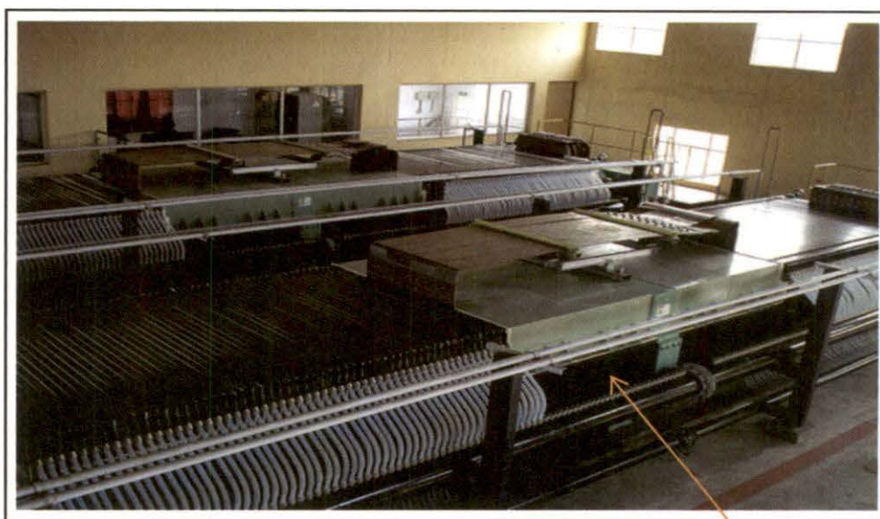
Electrolyser cells not installed
