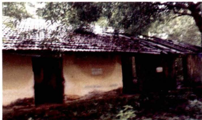
Dilapidated condition of leprosy hospital
