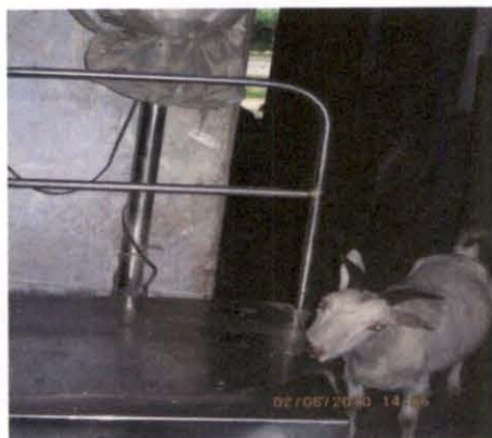
Easy accessibility of animals to Mancotta GPSS godown contributes to storage loss.
