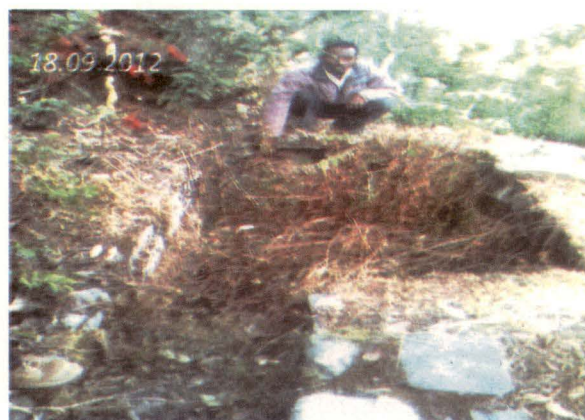
Non-functional Sarna Canal
