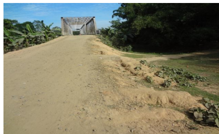
Incomplete approach and protection work of RCC bridge over Katakhal River on Srikona-Mohanpur Road (17-11-2013)
