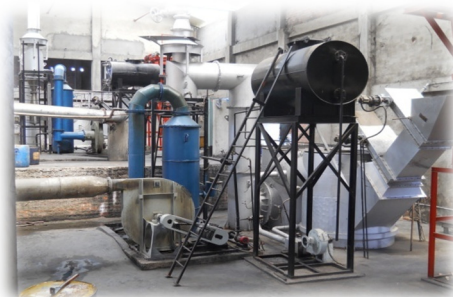
Incinerator at CBWTF
