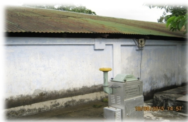
Air Monitoring station at Pragjyotish College, Santipur, Guwahati
