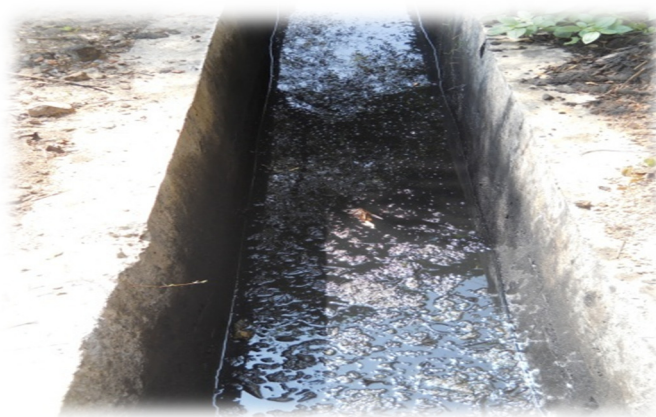
Drainage outlet at New Guwahati Diesel Locomotive Shed
