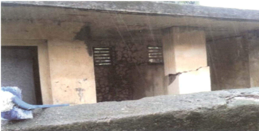
Picture-6: Toilet blocks of Upper Primary School, Varoli Talat, Valsad district, Gujarat, in damaged condition,
