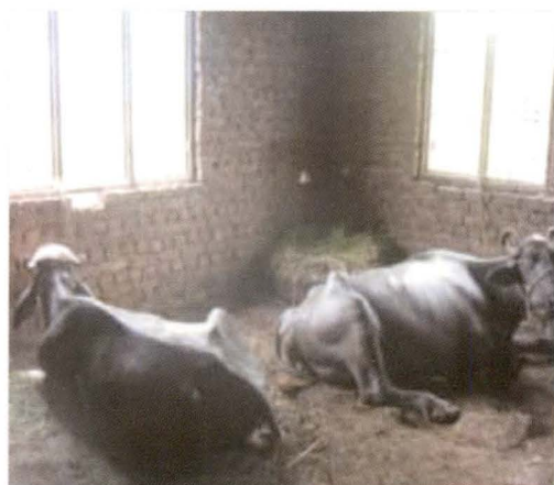
Picture-1: KGBV building (under Construction) Doongi, Rajouri, J&K being used by locals as cattle shed
