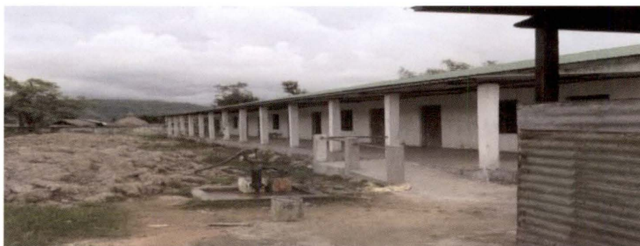
Picture-9 : Dokmoka Higher Secondary School, Karbi-Anglong, Assam – Building incomplete even after lapse of 12 months from due date of completion
