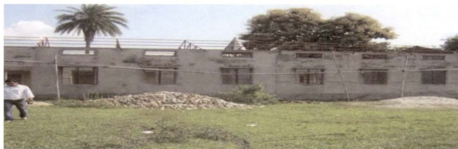
Picture-10 : Sankar Dev Mission high School, Udalguri, Assam – Building incomplete even after lapse of nine months from due date of completion
