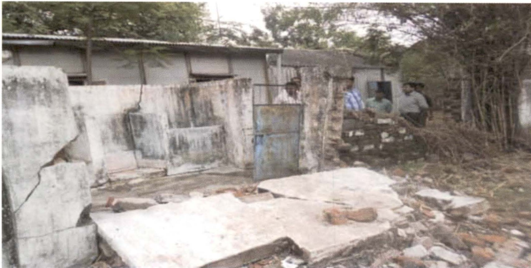
Picture-5: Damaged compound wall and girls' toilet of Primary School, Chandpuri Faliya, Dantol, Panchmahal, Gujarat
