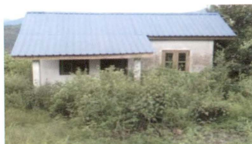
Picture-15: Unoccupied staff quarter surrounded by bushes at Maram PHC, Senapati District, Manipur
