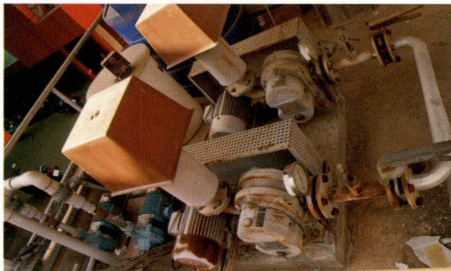
Parts of treatment plant got rusted
