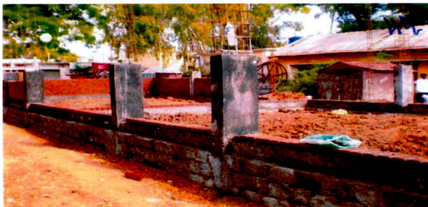
Incomplete work of Government Girl's High School, Molkalmuru
