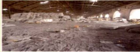
Cement dust at Salt Cotaurs Goods shed, Chennai
