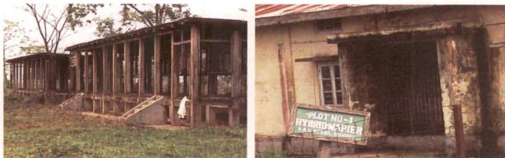
Dilapidated condition of live stock shed and building
