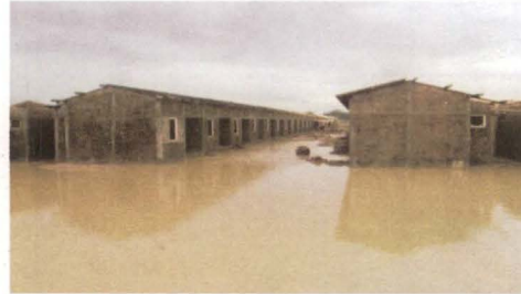
Water logging at IHSDP dwelling units at Karimganj (2 June 2010)
