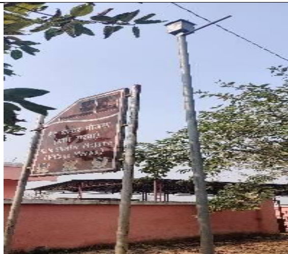
Picture A.2: Stolen Solar Panel of a Solar Street Light near Rain Shelter, Mojma, Bihar
