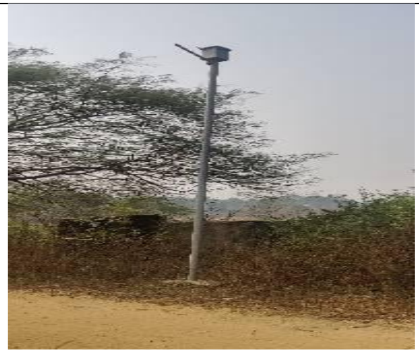
Picture A.3: Stolen Solar Panel of a Solar Street Light near Mini Cafeteria, Tankeshwar, Bihar
