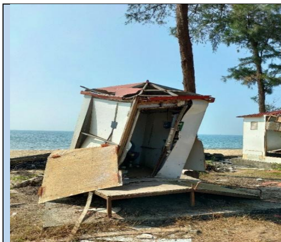
Picture 4.14: Damaged Gents' toilet (mobile toilet) at Keri, Goa
