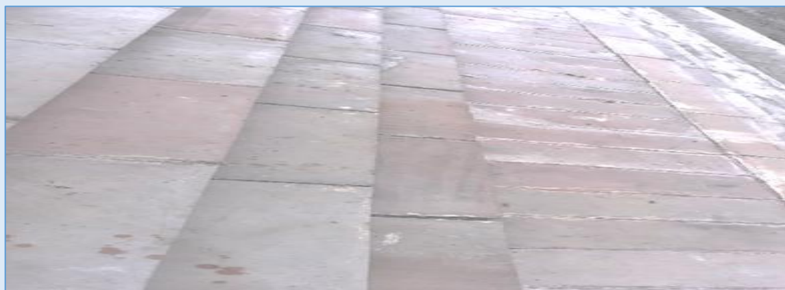
Picture 3.5: MS Clamps not fixed at Guptar Ghat, Ayodhya, U.P.
