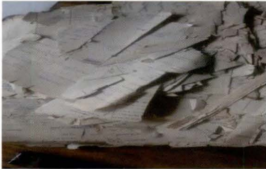
Condition of ledger of Karol Bagh Estate
