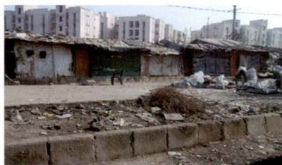
North Zone: Construction of Peripheral S.W. Drain & culverts in Sector G-7 & G-8
