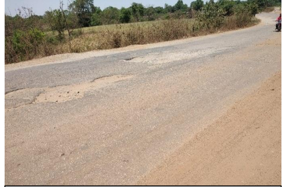
Picture No. 5.1.5: Poorly maintained Dharwad-Alnavar-Ramnagar road (May 2019).
