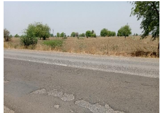
Picture No. 5.1.6: Poorly maintained Wagdhari-Ribbanapalli road (April 2019).
