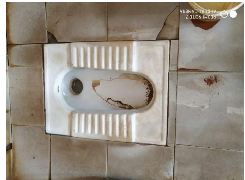
Picture No. 6.3.8: Sidlaghatta bus station – damaged toilet (July 2019).
