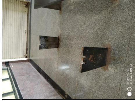
Picture No. 6.3.10: Sidlaghatta bu station – Missing bench for sitting (July 2019).
