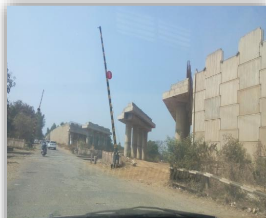
Picture No. 5.1.3: one of the three incomplete ROB at Chainage km 5+530 (April 2019).
