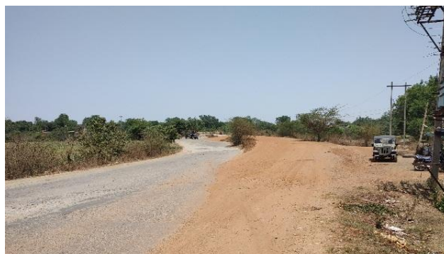
Picture No. 5.1.4: Incomplete approach road to ROB (April 2019).
