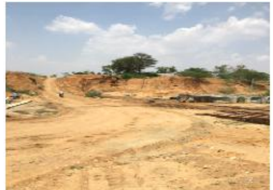
Picture No. 5.1.2: Incomplete bypass at Gowribidanur (May 2019).
