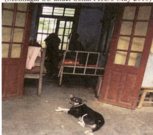
Photograph of unsecured maternal ward (Borkhola PHC/4 May 2010)
