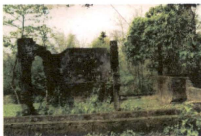
Damaged pump house and stilling tank of Udharbond ELIS, Bagerkona PC (Inoperative)/27 April 2010
