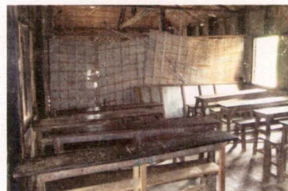
Dilapidated condition of a school/18 May 2010
