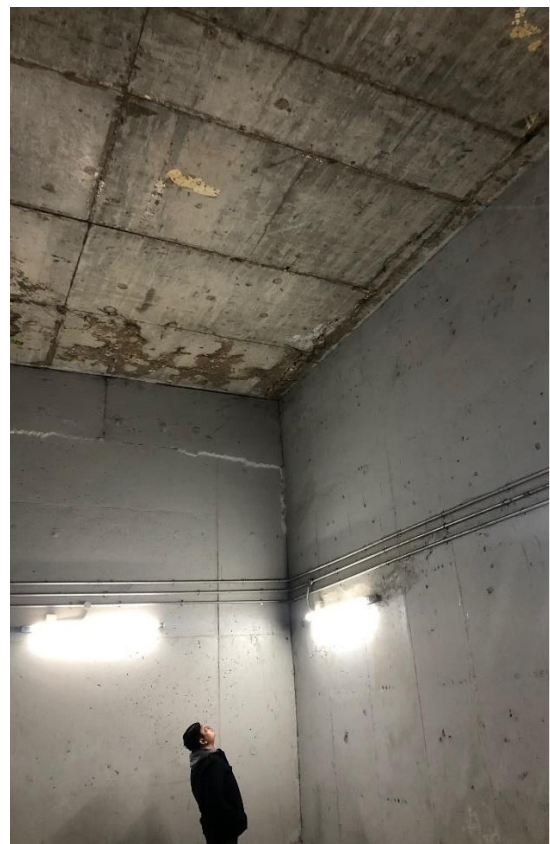
Honeycombing and poorly made formwork joints
