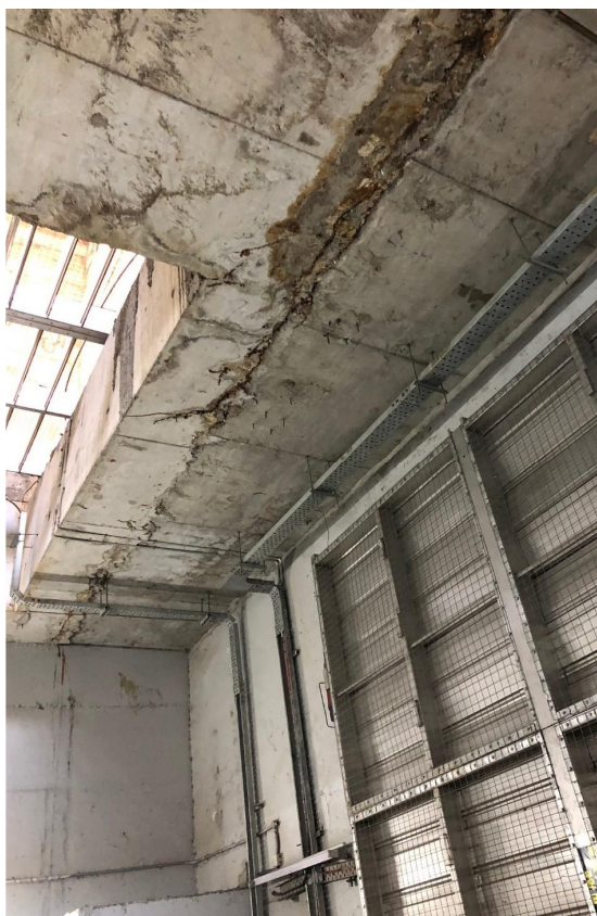
Honeycombing and bulged concrete surface
