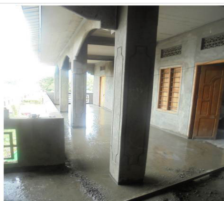
Cement flooring instead of tiles
