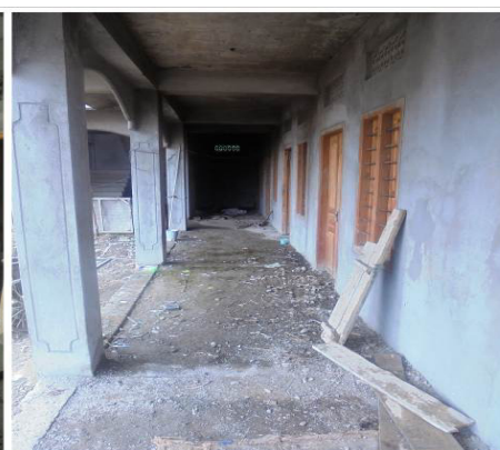
Internal electrification not installed
