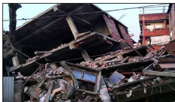
Damage at a residential building at Dewlahlane, Imphal East District
