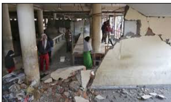
Damage at Ima Market, Imphal West District
