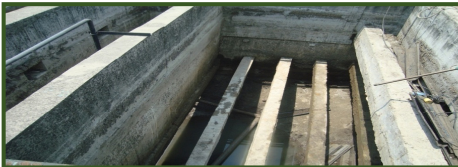
Non-operational STP of OMAXE Reveria Infrastructure, Rudrapur, Uttarakhand
