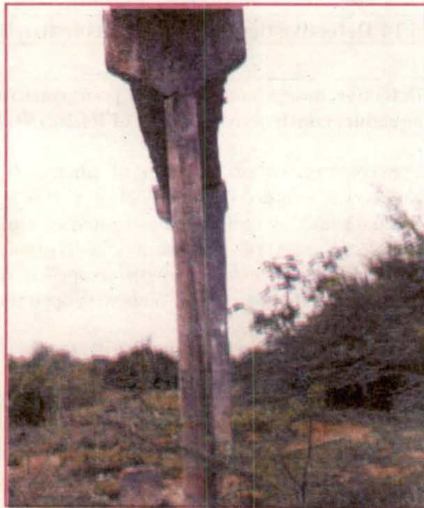
Severe honey combed concrete and non verticality of piers
