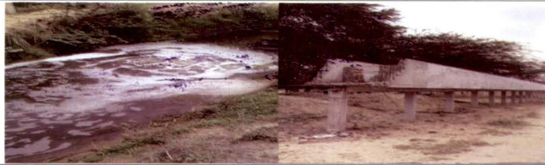
Incomplete sewerage scheme Ellenabad due to abandoned effluent channel (April 2016)
