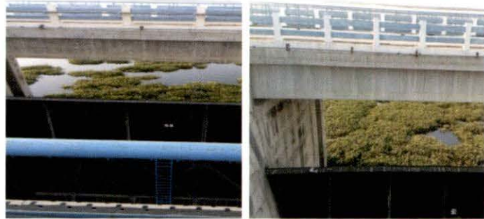
Echhornia Plant growth in front of gate number 3 of the Gosikhurd Reservoir
