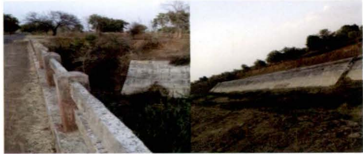
Skidding of Retaining wall at RD 31020 m
