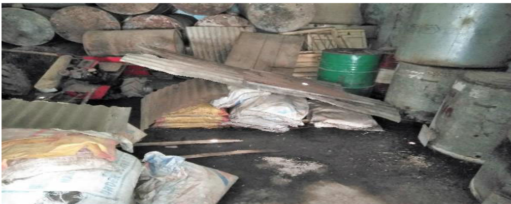
Figure 2.1.6: Damp seed godown of BSF Jalangi Rain water visible on the floor
