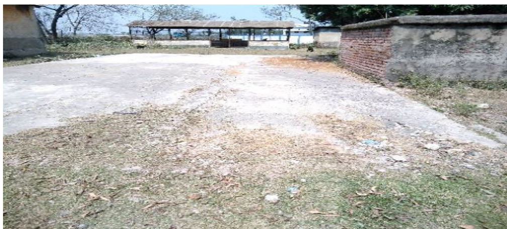
Figure 2.1.1: Damaged open threshing floor of BSF Kaliaganj
