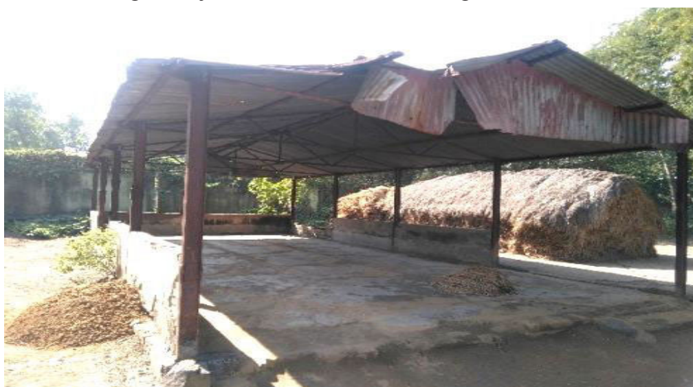
Figure 2.1.2: Damaged covered threshing floor of SARF Saltora
