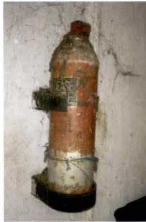
Picture 6.1: Poorly maintained fire extinguishers in Brilliant Ice Plant, West Hill, Kozhikode (18 May 2017)
