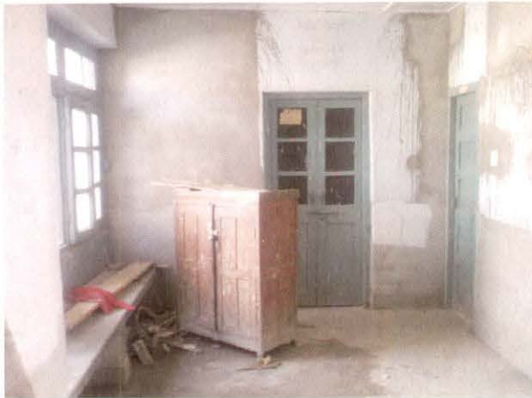
Condition of Operation Theatre at CHC, Kotli (June 2010)
