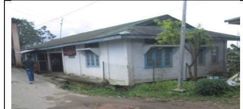
Old Court Rooms at Mon in dilapidated condition
