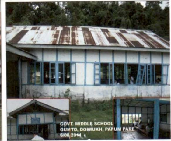
Sub-standard School building-GMS, Gumto, Doimukh
