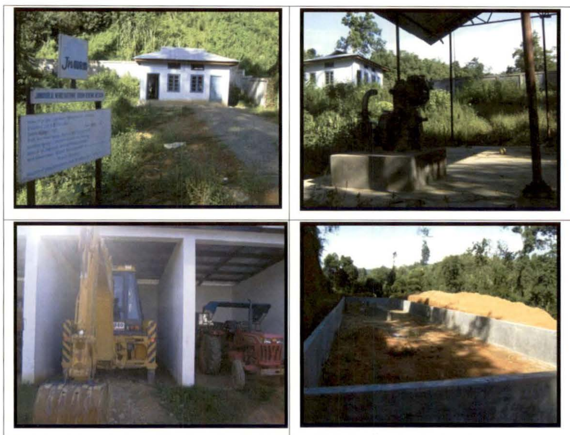
Photographs of various stages of construction of solid waste management at Jairampur.
