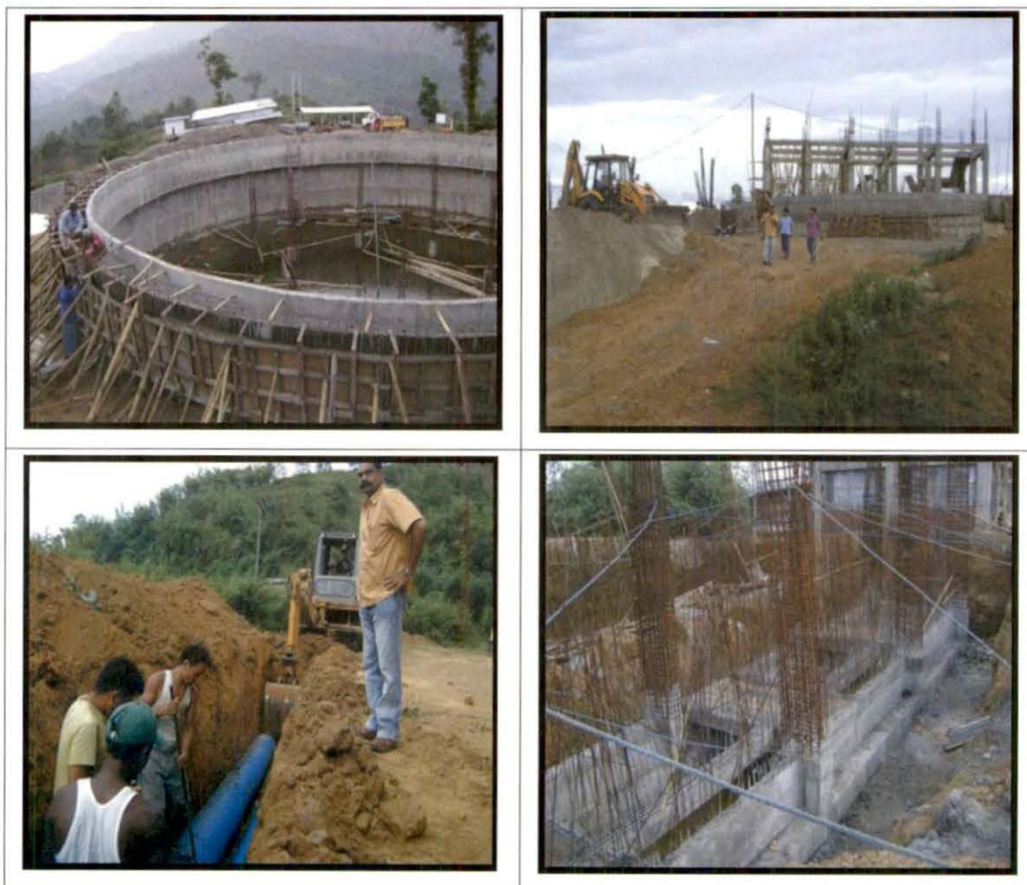
Different stages of construction activity in respect of the project 'Augmentation of Water Supply at Mission City Itanagar'
