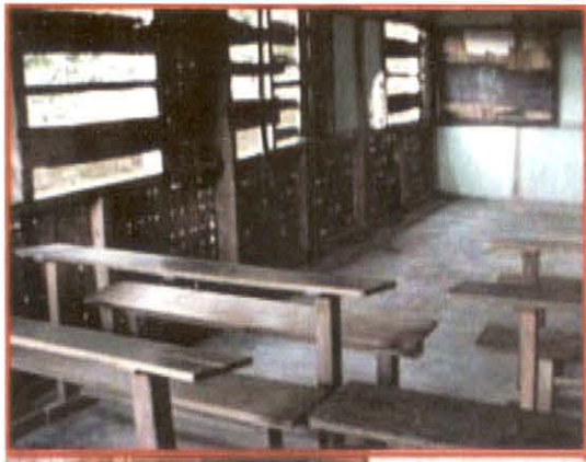
Condition of classroom in Hr.Sec.School (U/Primary section), Balijan
