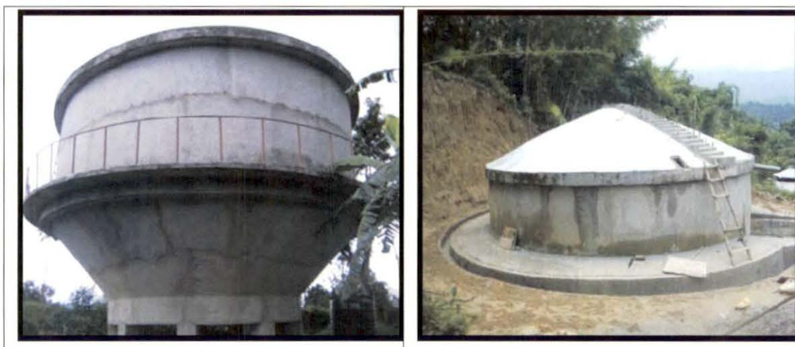
Photographs completed storage tanks lying unused due to incompleteness of work intake point etc in the project 'Augmentation of Water Supply at Mission City Itanagar'
