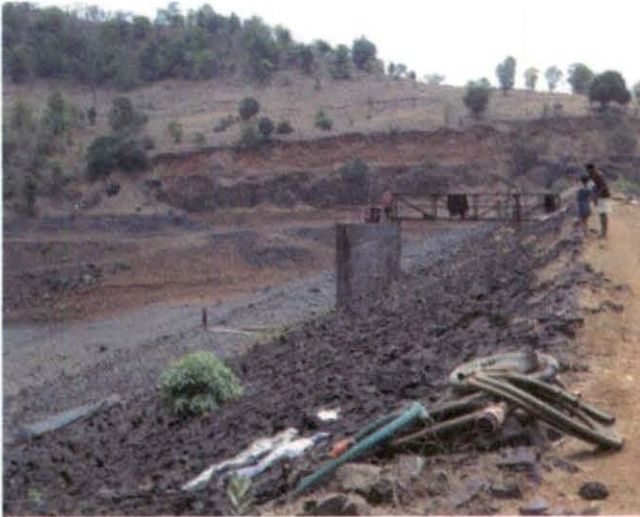
Tangar (leakage at dam flank)
