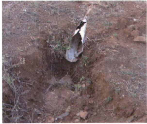
Tulyachapada (breakage of underground pipeline)
