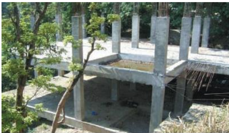
Photograph dated 4 June 2012 of construction of ITI building at Shimla lying suspended.
