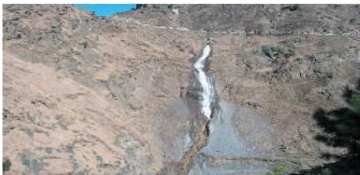
Photograph dated 3 April 2012 of Hydro Electric Project Chirchind-I (Chamba District): Open Spillway without MS Pipe
