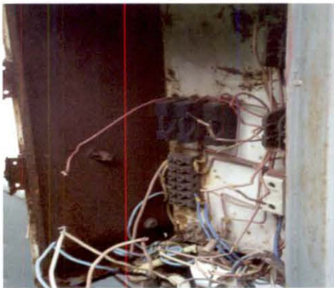
Electrical Panels of the Lock Gate
