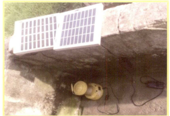
Solar panels - sole source of power in the camps
