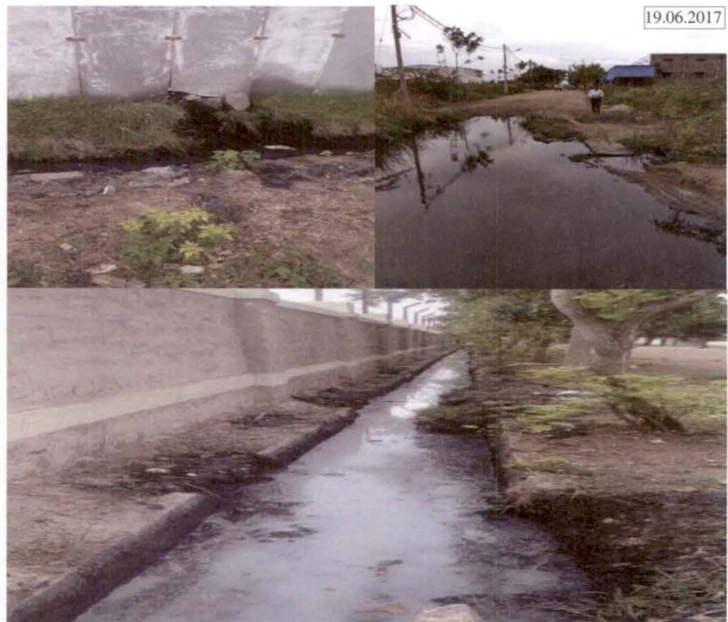
Photograph 2.1: Industrial effluents flowing out in open drainage at Mundaragi
