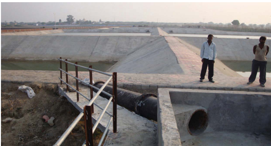
Incomplete STP 2.76 mld (WSP technique) at Mathura
