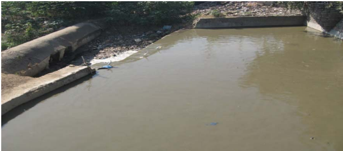
Blocked I&D works at Afzal Sagar I&D in Hyderabad, Andhra Pradesh
