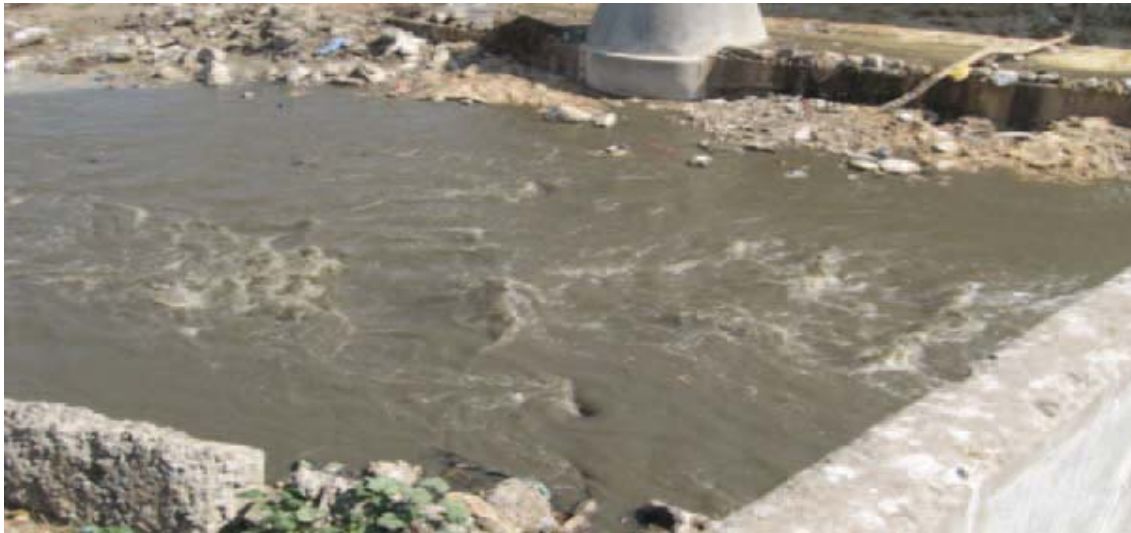
Blocked I&D at Murinala in Hyderabad
