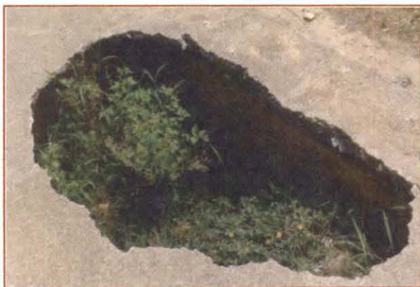
Picture 4.7: Bad condition of Pandivillai Road
