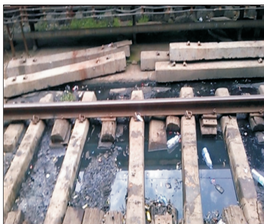
Out sourced arrangements for cleaning Platform line of Mumbai central (A-1) station (WR)
