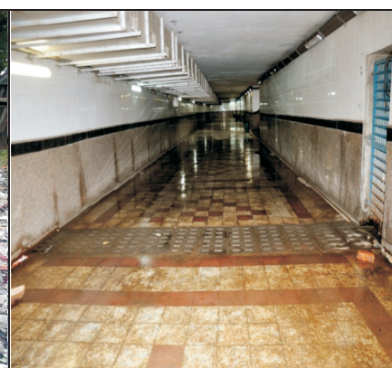
Water logging in Subway/Underpass at Kolkata station of A category (ER)
