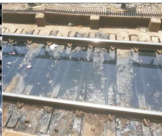
Poor cleanliness of line on PF No. 2 & 3 of Vadodara A-1 station (WR)
