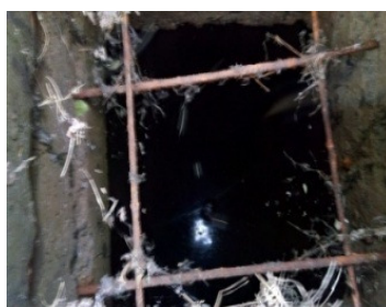
Water logged structure at RPS Infrastructure, Faridabad
