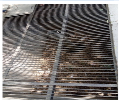
Leaves and mud in RWH structure at Food Corporation of India, Faridabad
