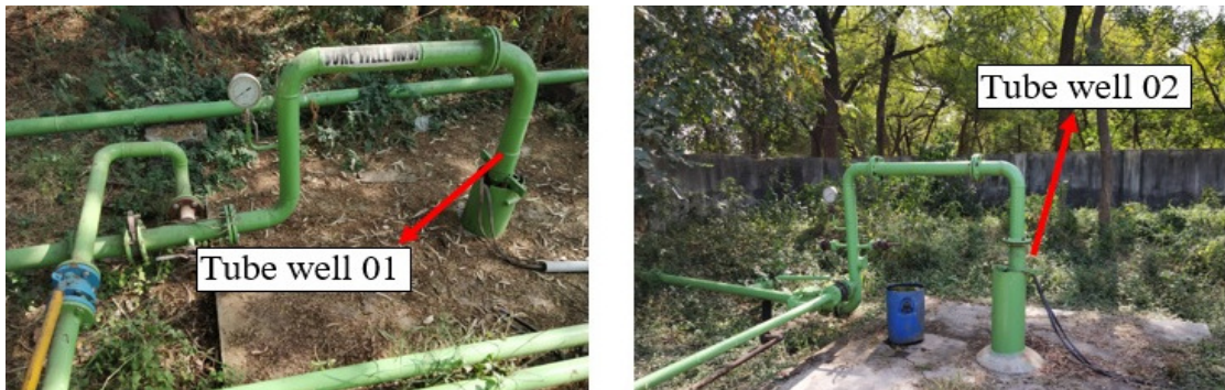
Tube wells being operated without installing water flow meter
