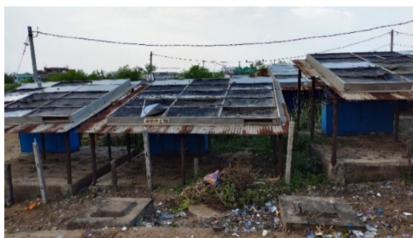
Fig. 34: Damaged Solar Panels at Nolia Nuagaon
