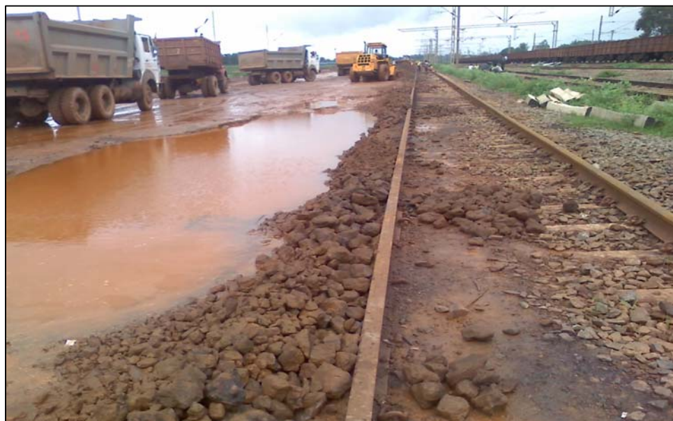
Broken concrete basement at Jagdalpur goods shed
