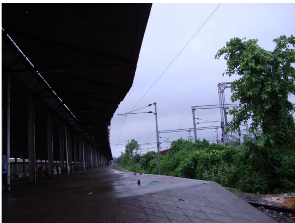
Chipped platform shed - Cuttack goods shed
