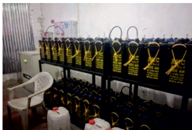
Solar batteries stored at Server room in Lawngtlai District Court
