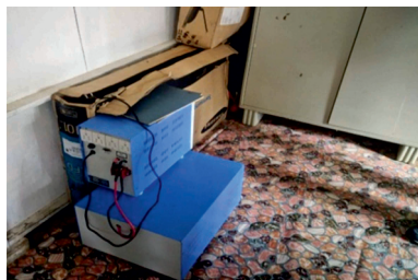
1 KV UPS, Samsung LED at Aizawl Central Jail
