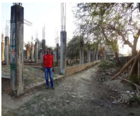
Four storey RCC building of General Nursing Midwifery (GNM) School-cum-Hostel at Nagaon (30.06.2016)
