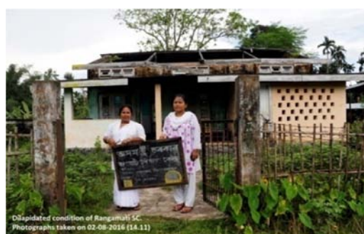
Dilapidated condition of Rangamati SC, Kamrup(R) district (02.06.2016)
