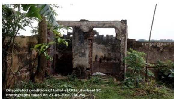
Dilapidated condition of toilet at Uttar Borbil SC, Karbi Anglong district (27.05.2016)
