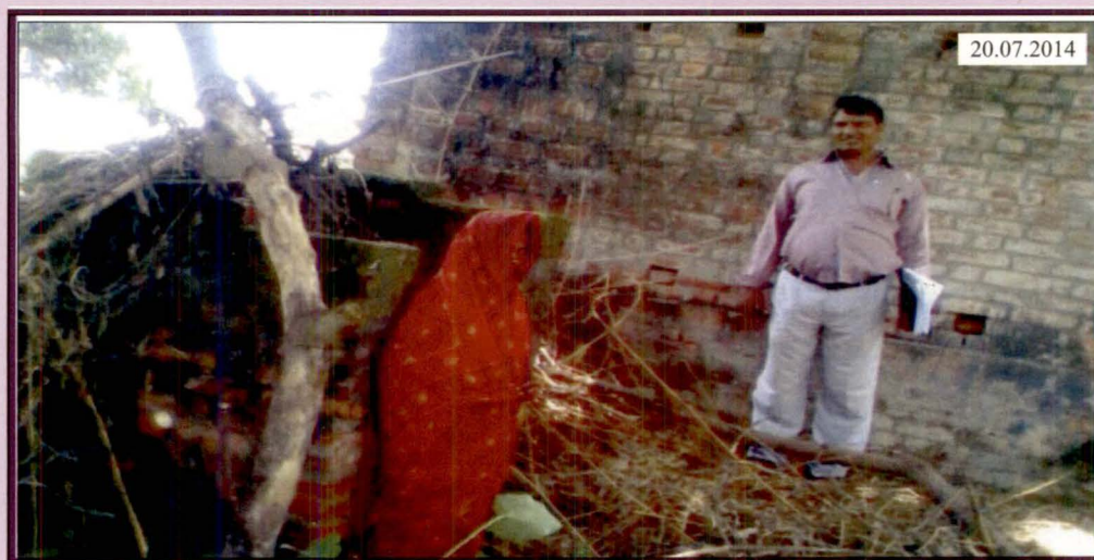
(Broken IHHL of a beneficiary of GP, Dhavarkan, block- Bhatpar Rani, Deoria)
