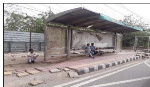
Figure 14: Poorly maintained BQSS with broken flooring
