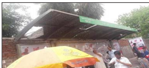
Figure 15: BQS with broken roof
