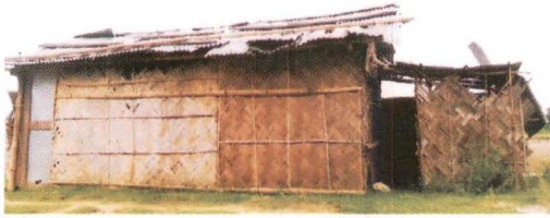
Dilapidated temporary shed at "Balupara FIS" site (21 May 2013)
