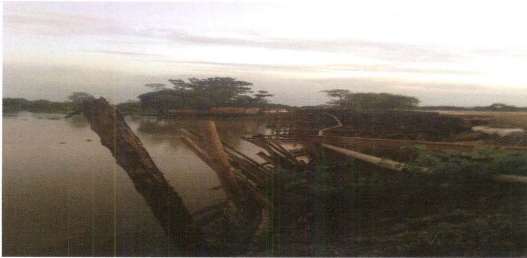
Present condition of construction site, with dilapidated condition of existing SPT bridge (25 August 2011)
