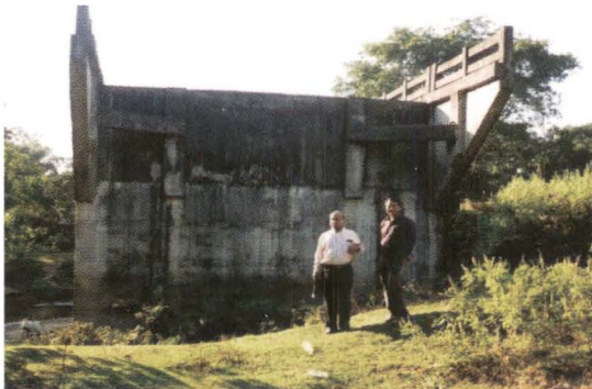
Bridge proper without any approach and protection work on Simaluguri side. (November 2012)
