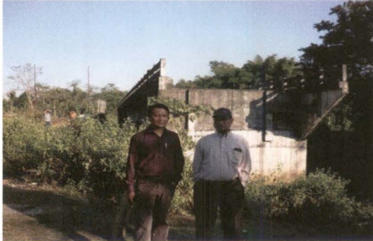
Bridge proper without any approach and protection work on Sonari side. (November 2012)
