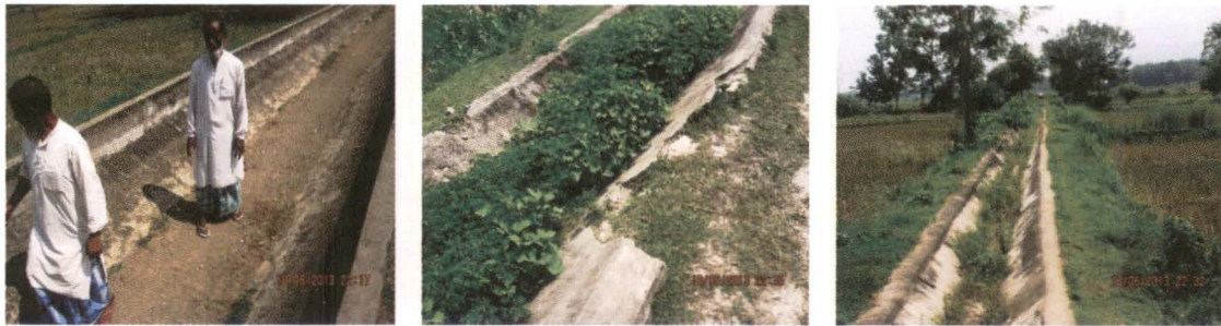
Damaged and Idle Main as well as Branch Canals under the schemes (18 June 2013)
