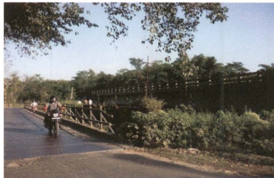
Existing steel bridge constructed by ONGC on up stream of the bridge. (November 2012)
