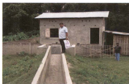
Incomplete pump house of LIS from River Tuni in Komargaon Area, Majuli (15-06-2013)
