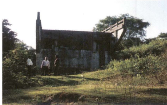
Incomplete earth work for bridge approach without any retaining wall and protection work on Simaluguri side. (November 2012)
