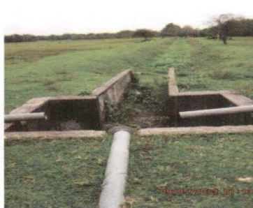
Discharge point of lift point 2 (9 May 2013)
