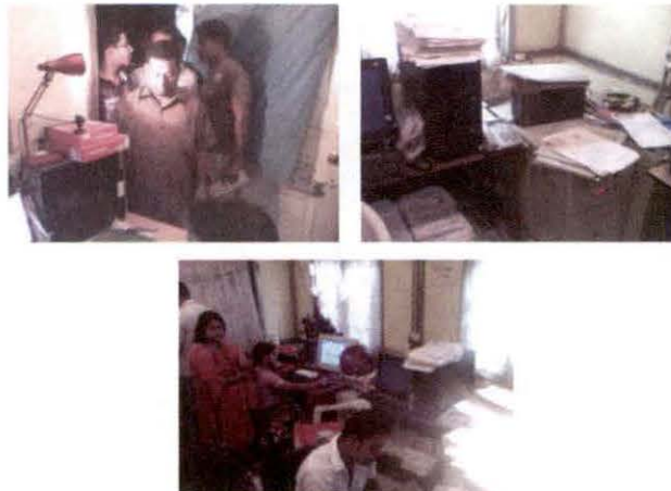
Pictures of server room of DTO, Nagaon depicting congestion, unrestricted entry and stocking of papers on the servers, UPS and batteries.
