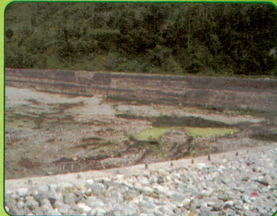
Incomplete work of Solid Waste Management at Shipchu (work was started four years back)
