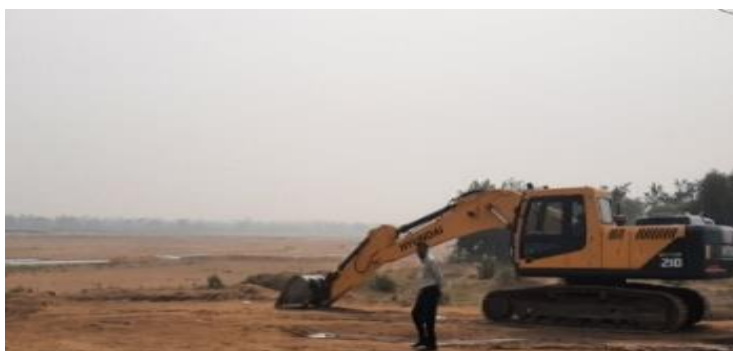
Figure- 4.2: Use of Poclain machines at sites (Balodabazar District, date of image: January 2021)
