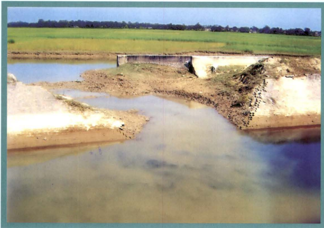
Breakage in Saharghat Branch Canal at tail end of WKMC
