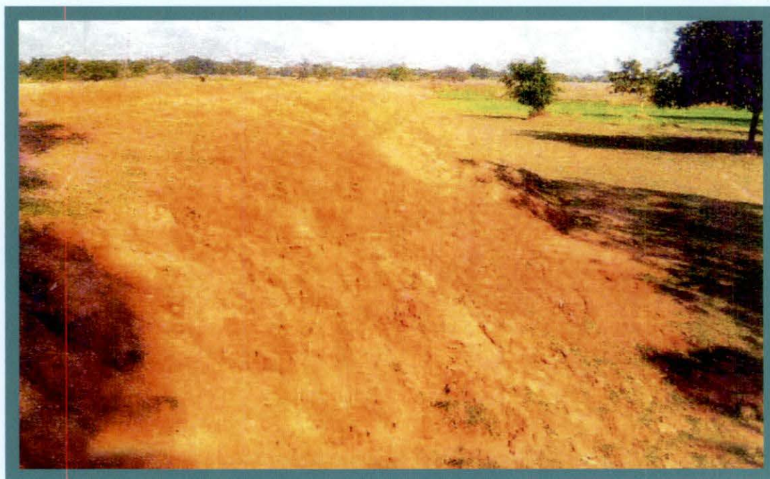
Incomplete work in Left Main Canal of Panchkero Reservoir Project
