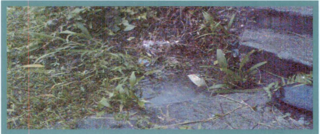
MI Project Damala Gaon – Non-visible channel due to non-maintenance
