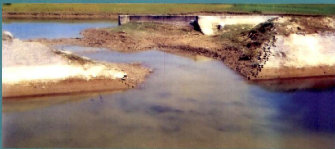
Western Kosi - Bihar : Breakage in Saharghat Branch Canal
