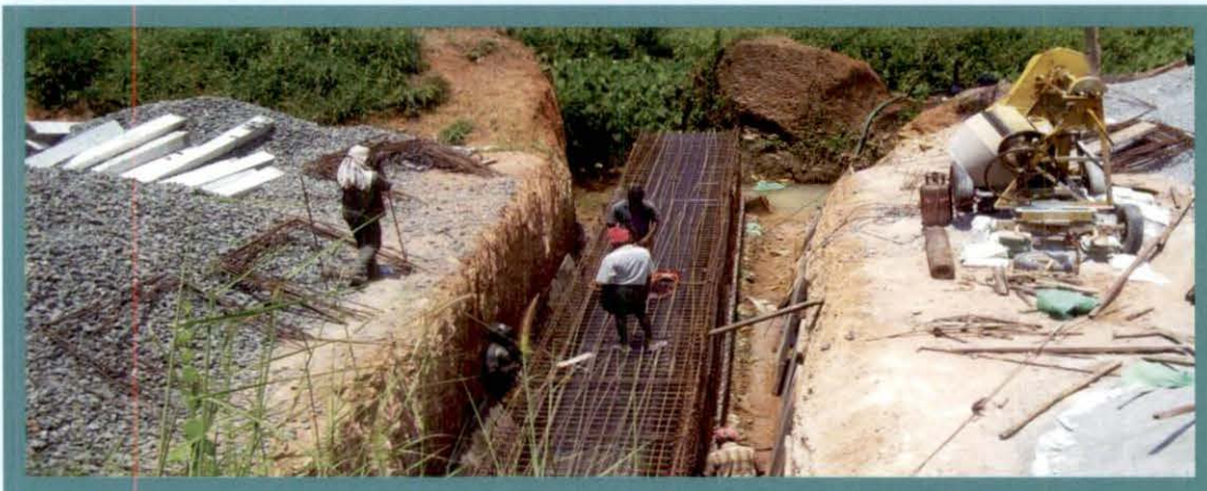
Bottleneck in work of Railway Portion of Poovattoor Distributary of Kallada Irrigation Project
