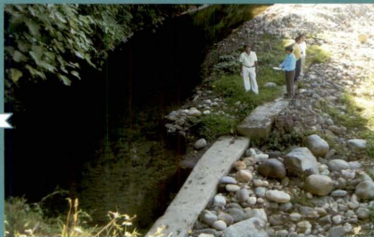
Completely damaged headwork at "Renovation of Headwork of Gagur MI Project" at Niglok, Pasighat Division
