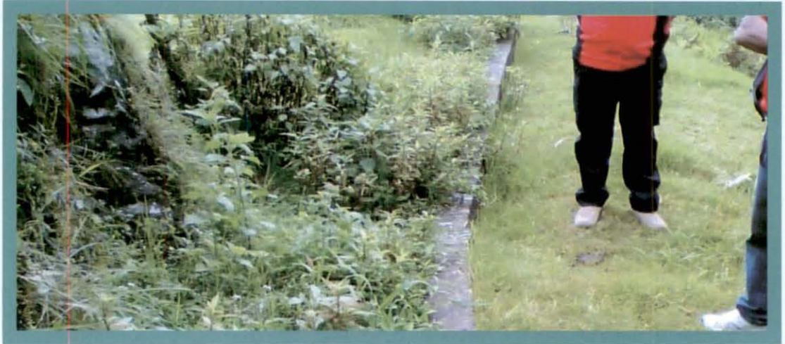
MI Project at Ramathang – Poor condition of the MI channel due to non-maintenance
