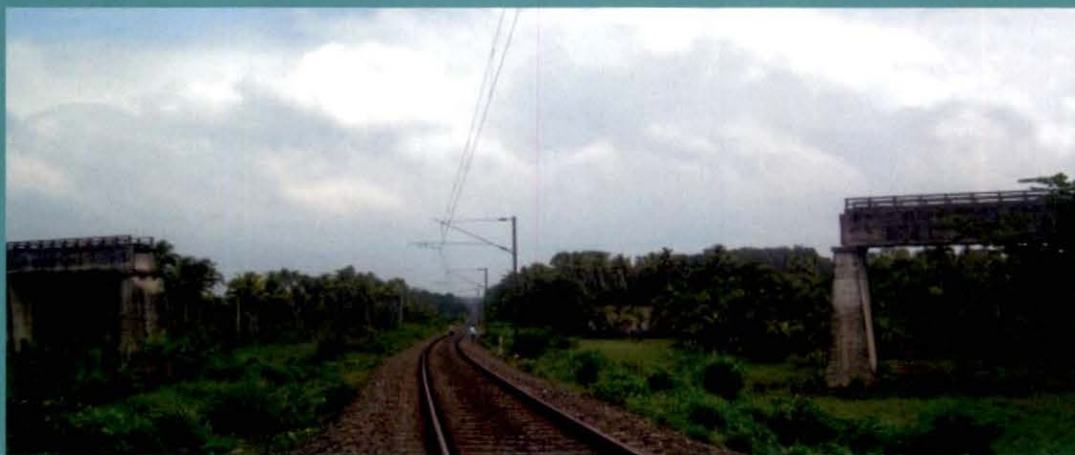
Muvattupuzha Irrigation Project– Kerala : Ezhuthonipadam Acqueduct - Bottleneck work in the Railway portion – Work yet to be arranged
