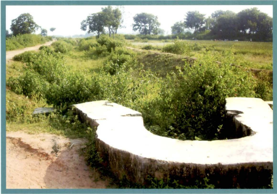
No water and need for bush clearing at Chainage 319 km of Tapkara Project
