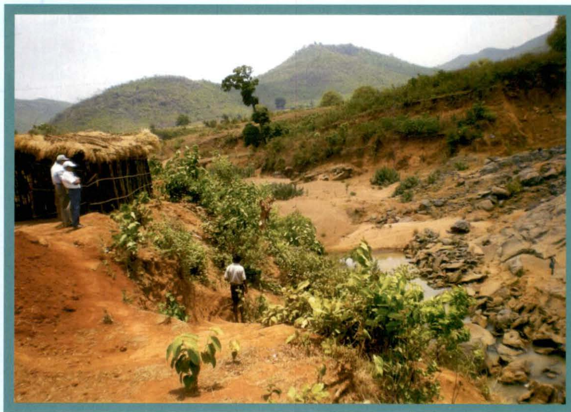
Telengiri irrigation Project – Abandoned site of spillway
