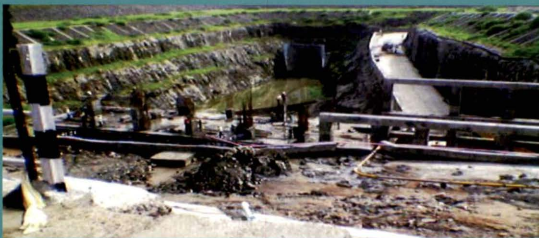
Indira Sagar Project (Canal) – Madhya Pradesh : Punasa Exit Channel – Work in Progress
