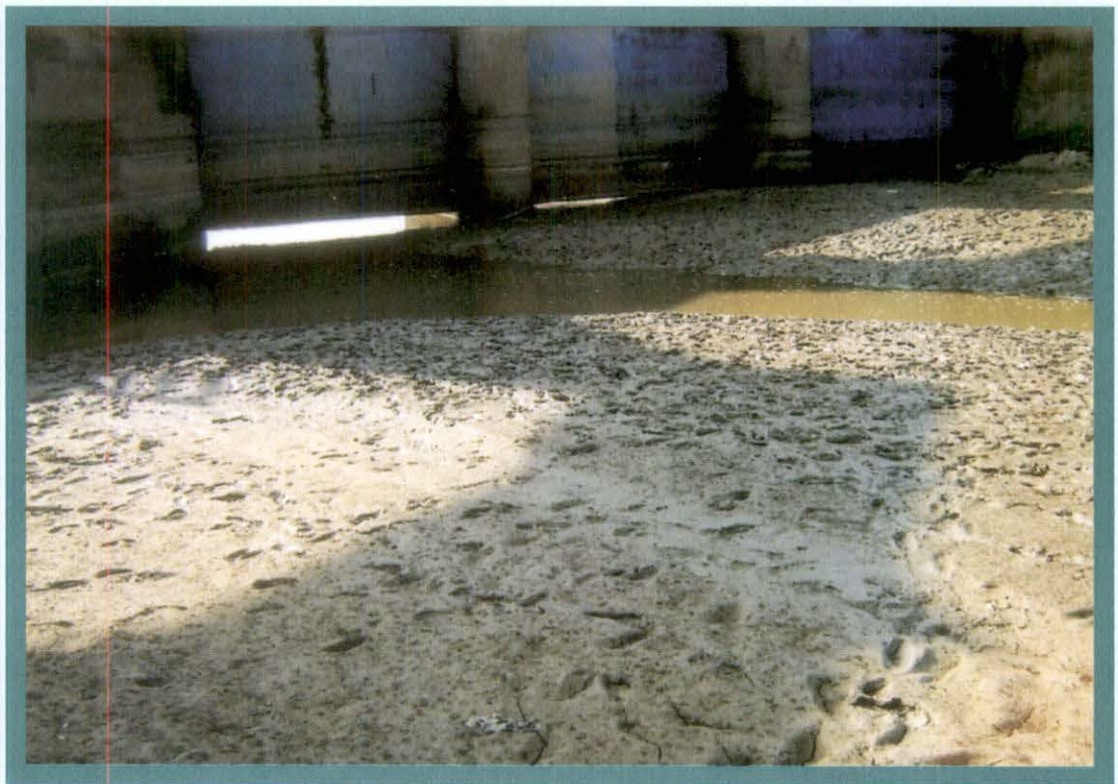
Siltation in upstream of Western Kosi Main Canal (WKMC) at RD 55 Km
