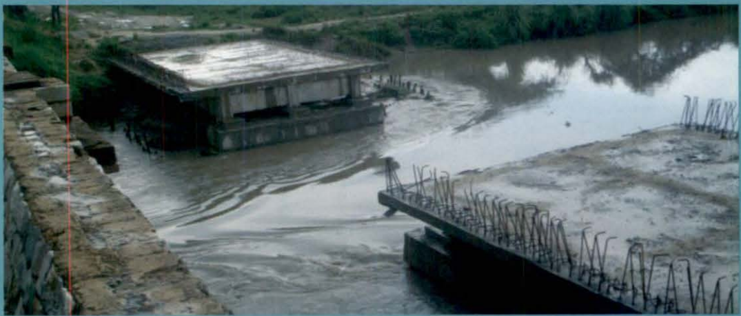
Agra Canal Project – Uttar Pradesh : Incomplete bridge at Chhajunagar (despite the fact that the project was declared as completed)
