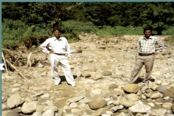
Non-existent headwork at M1 Project in Mane Village, Itanagar Division
