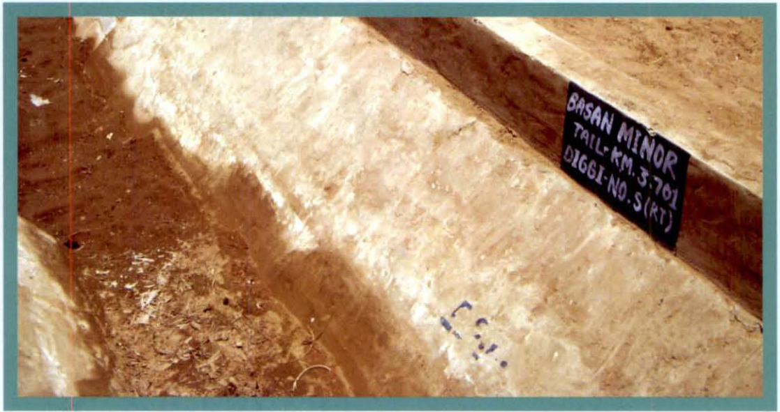
Narmada Canal Project – Incomplete work in the Inlet of Diggi No.5 Basan Minor at tail 3.701 km – Vank Distributary
