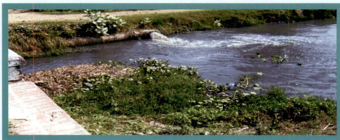
Discharge of Sullage/Polluted water at RD 58500 metre of Chheharata Distributary of Upper Bari Doab Canal (UBDC)
