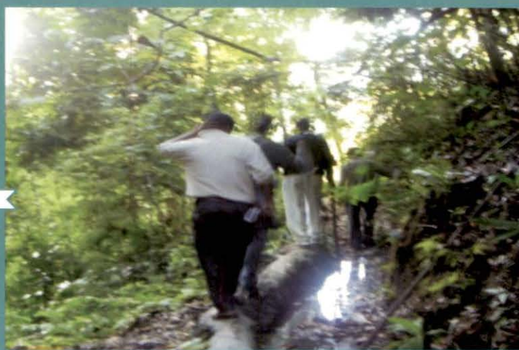
Damaged earthen canal at M1 Project from Teer Stream to Hoya Happa at Yachuli Village, Ziro Division
