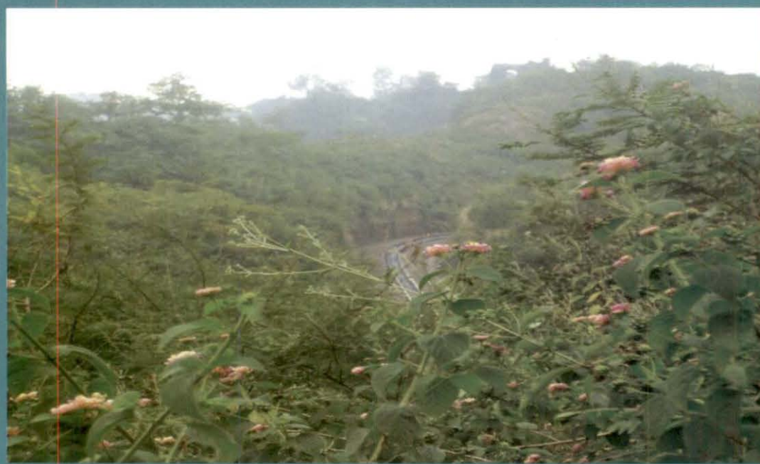
Work held up due to railway land falling within canal alignment
