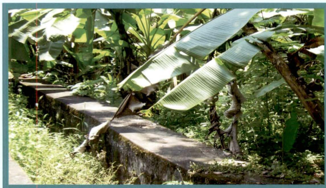
Pulamon Distributary of Kallada Irrigation Project – Canal filled with grass and plantations on the banks
