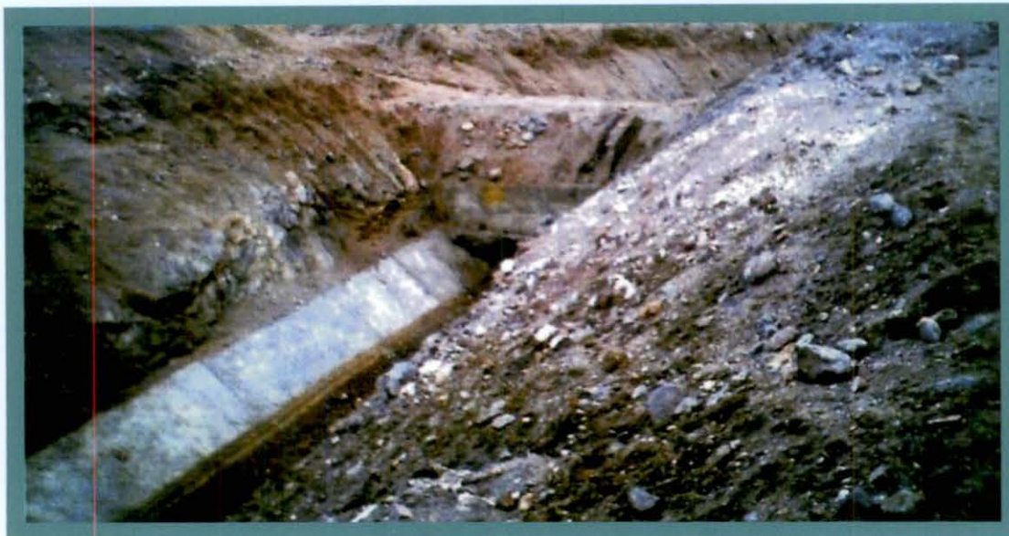
Bottleneck in tail end of Almatti Left Bank Canal of Upper Krishna Project Stage-II
