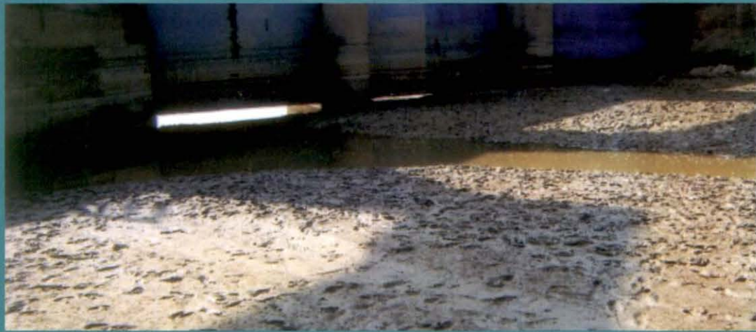
Western Kosi Main Canal- Bihar : Siltation in upstream
