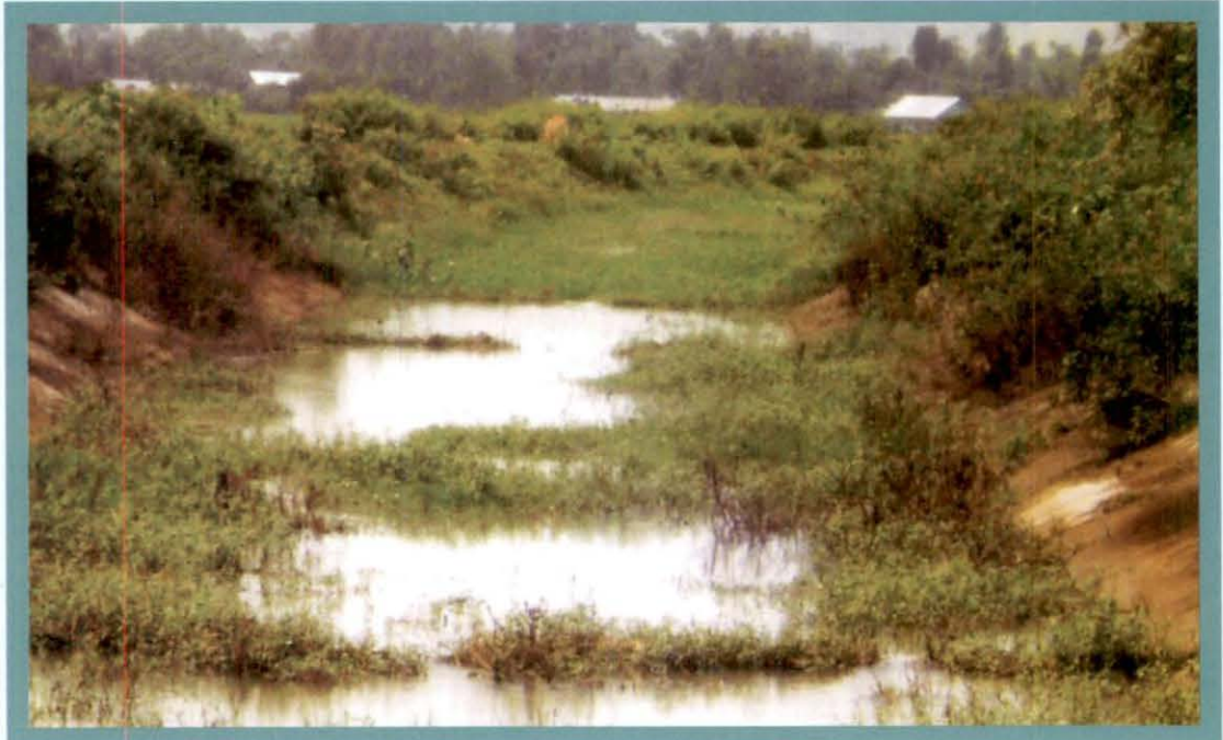
Thoubal Multipurpose Project - Siltation & shrubs/ weeds in canal
