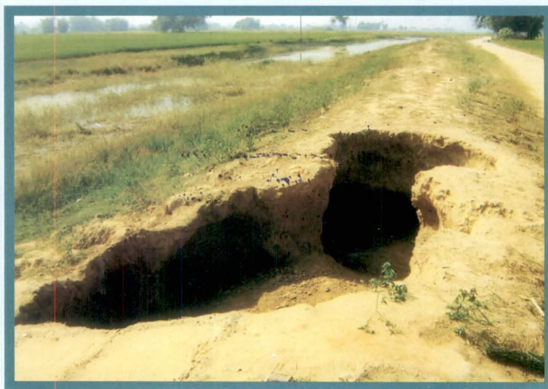
Damaged embankment of Gerua Reservoir Scheme
