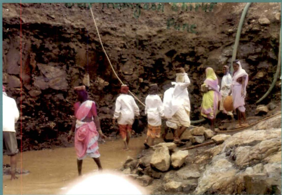
KT Weir at Inamgaon – Non-completion of work despite availability of sufficient funds
