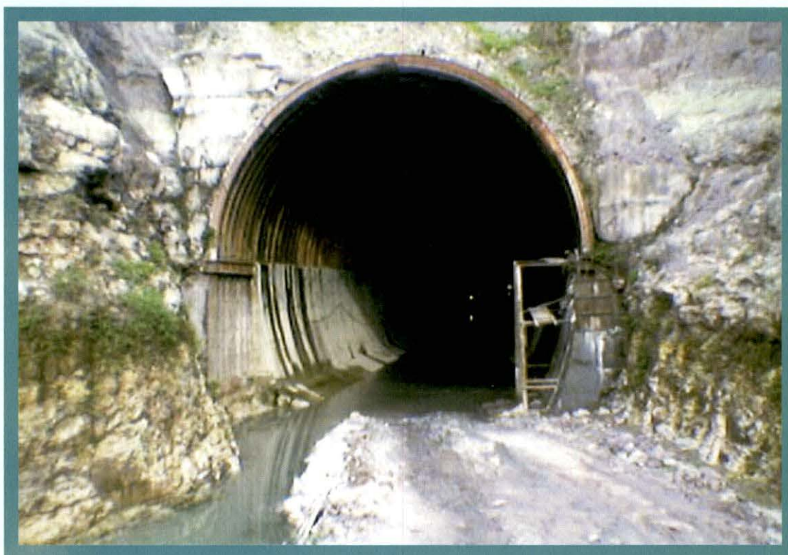
Incomplete tunnel work at road 33 to 35 km of Bargi Diversion Project – Ph-I
