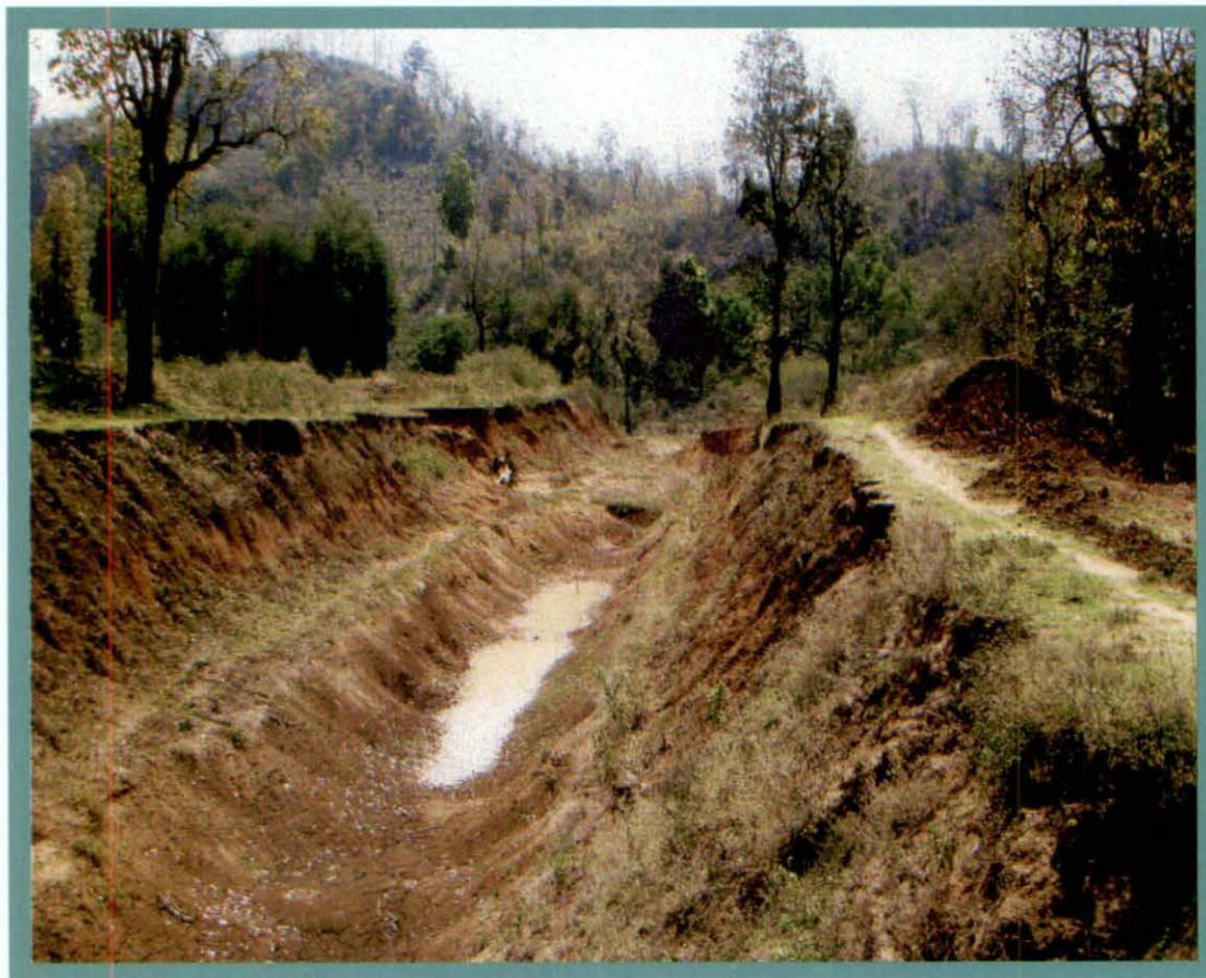
Doraguda MI Project – Incomplete Head reach canal from RD 00 metre to 1250 metre
