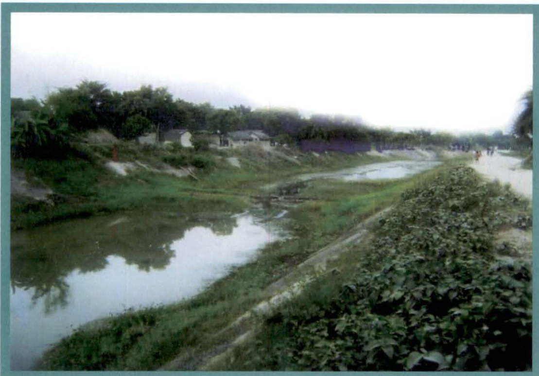
Siltation and vegetation in WKMC at RD 135.45 Km
