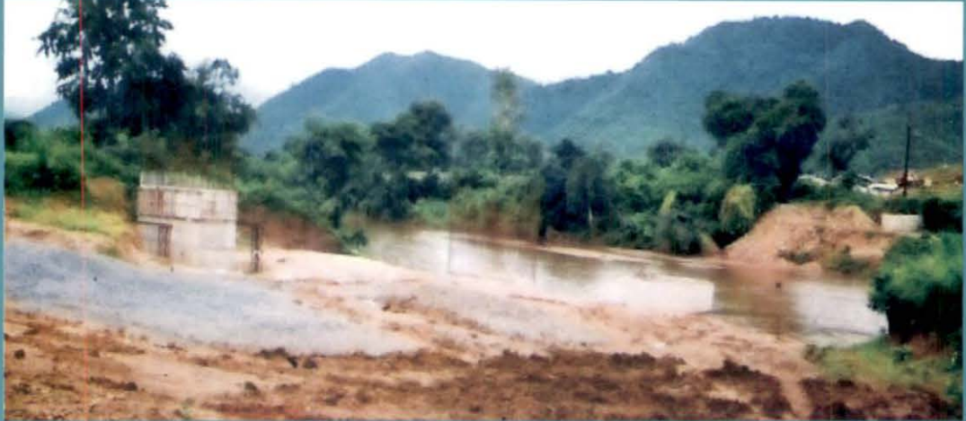
Upper Indravati Irrigation Project – Orissa : Syphon Aquaduct over river Sagada at RD 2820 M of RBMC remained incomplete due to non finalization of design
