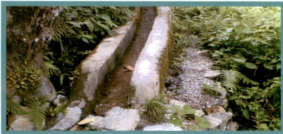
MI Project at Khanikhola to Pradhangaon – Defunct MI Channel
