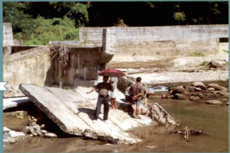
Damaged headwork at MI Projection Kanabung Village, Itanagar Division
