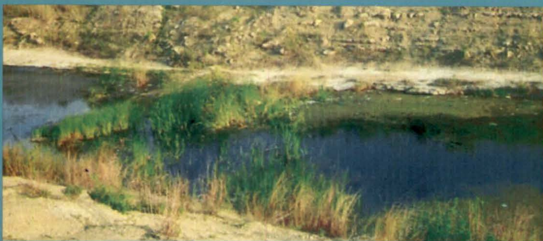
Right Bank Canal (RBC) of Rengali Irrigation Project – Orissa : Failure of slope and slippage of embankments at RD 31.55 to 34.24 km
