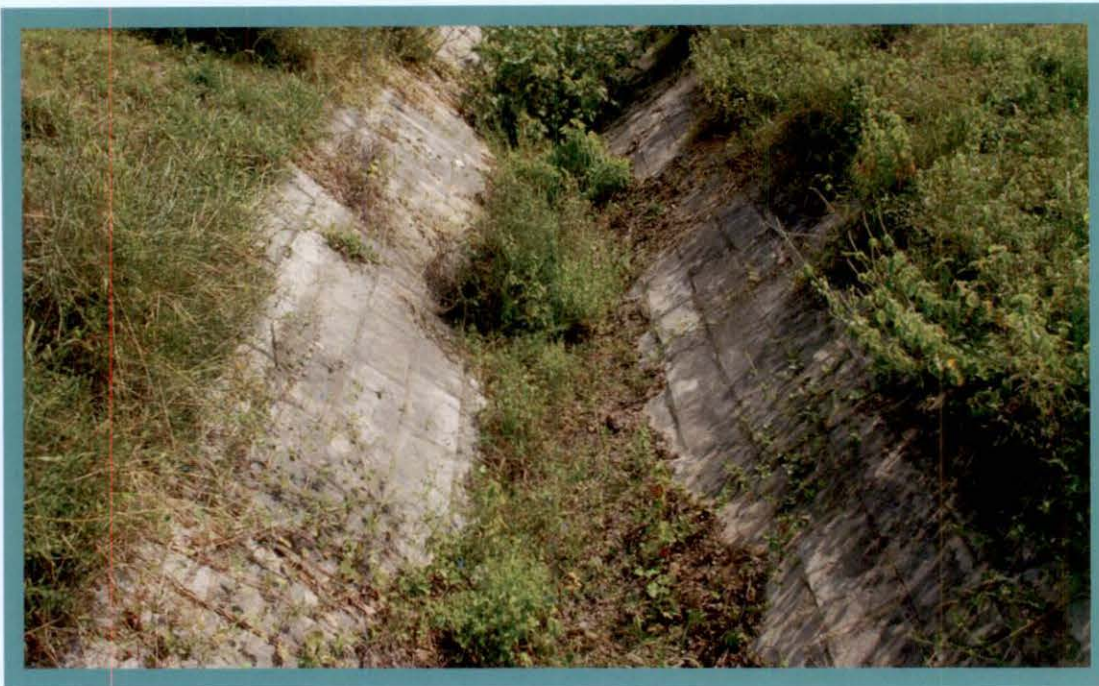
Mukteshwar Project-Dry canal with Weeds and Siltation
