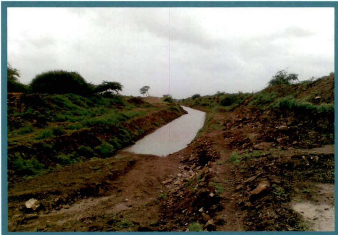
Bhadar-II Project- Incomplete canal
