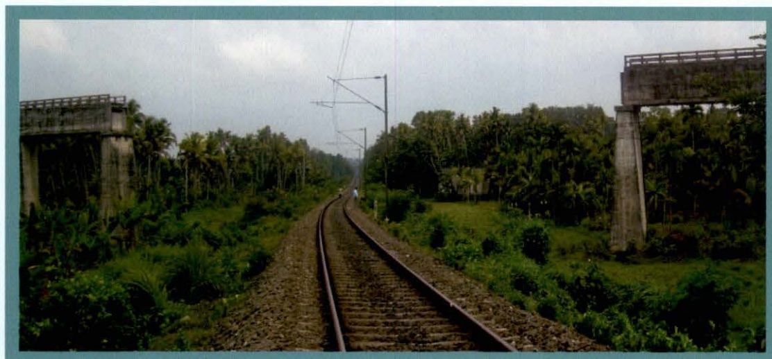
Non-initiation of work on Ezuthonipadam Aquaduct over Railway Line in Muvattupuzha Irrigation Project
