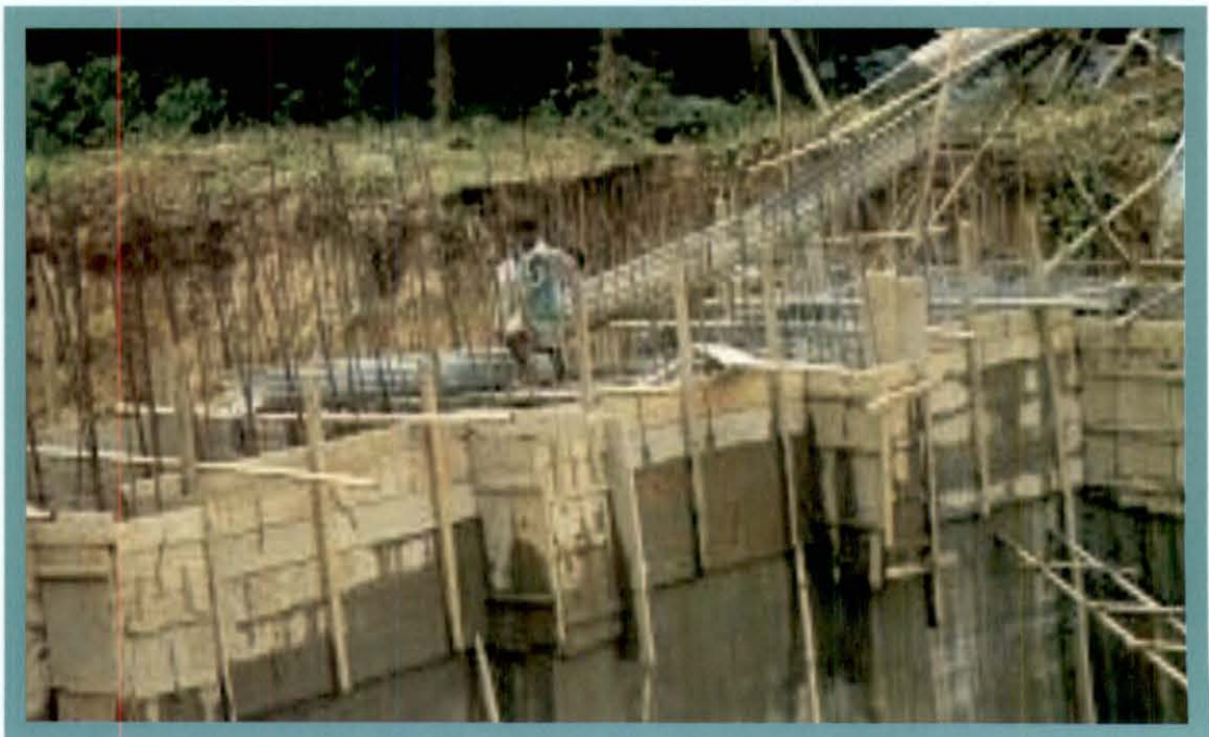
Awokupughoki MI Project – Work in progress in July 2008, despite the project being declared as completed in January 2008
