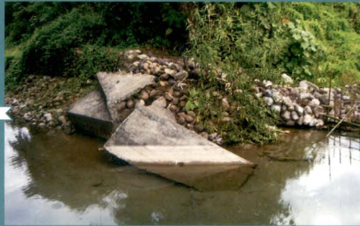
Damaged headwork at Eme Garsing (M) & Rangkop Area at Sigar, Pasighat Division
