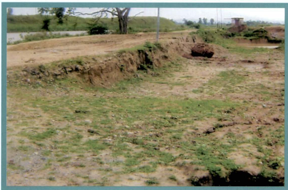
Incomplete WPLC under SCMP
