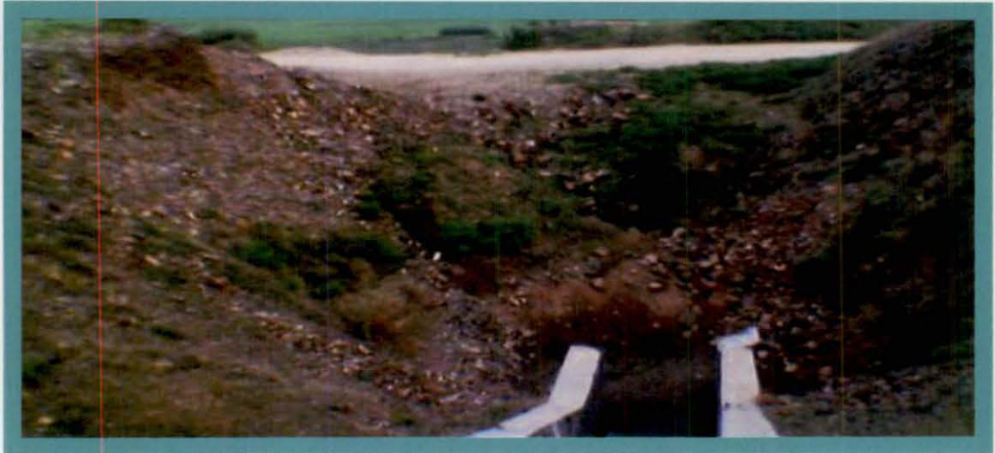
Bansagar Project (Unit-II –Canal) – Madhya Pradesh : Sihawal canal - Incomplete structure at Rd km 42
