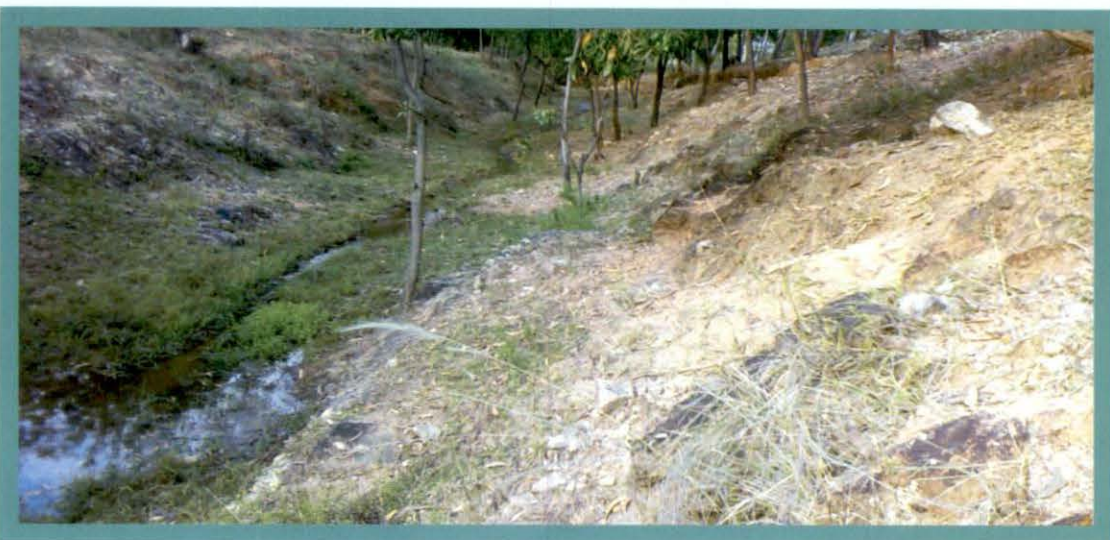
At Ch. 198.00m no canal water at RBMC of HIS in Purulia District was available due to rocky zone. (The water in picture is rain water)
