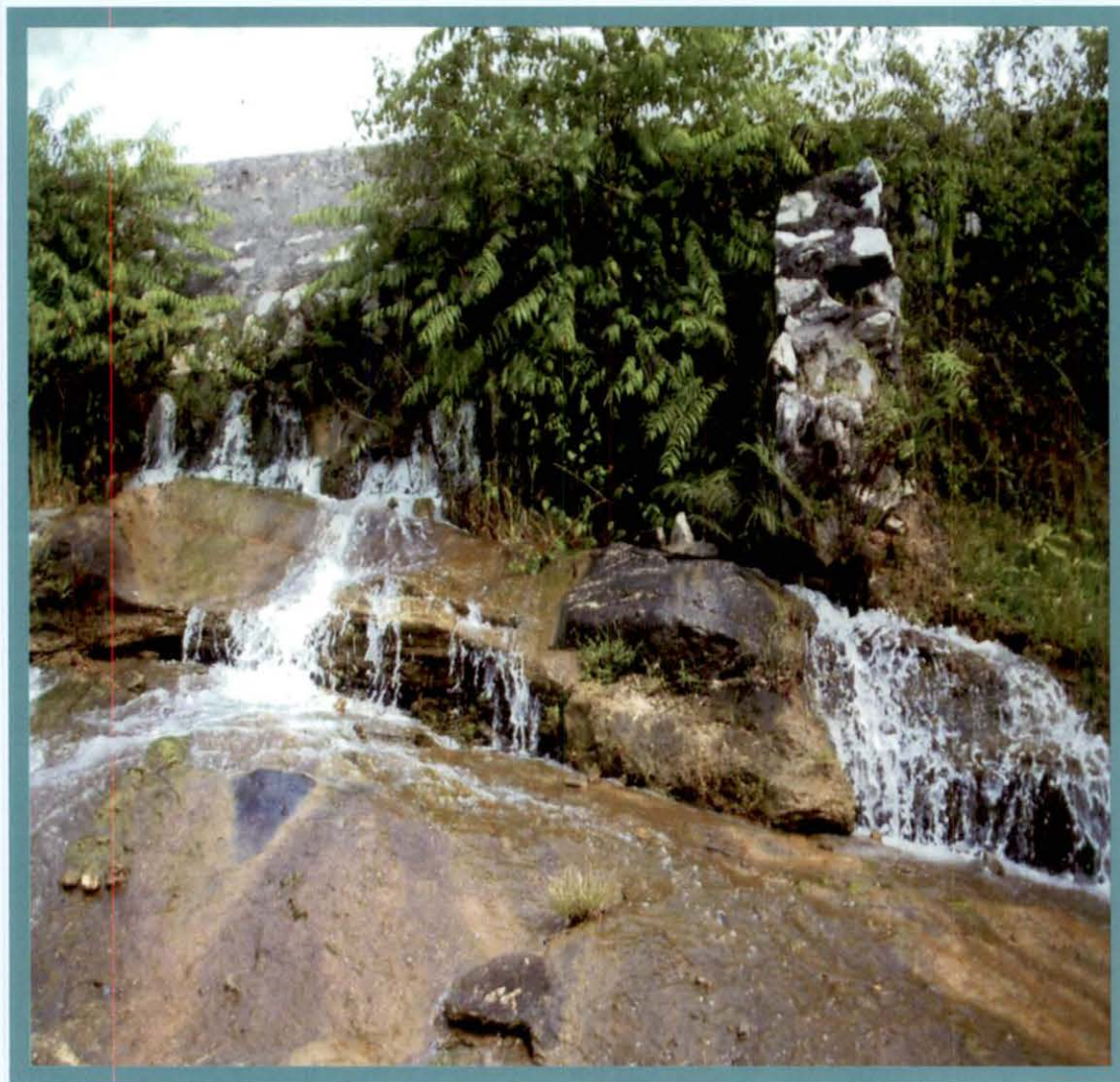
Damage of canal boulder masonry wall at Chainage 11 km of Tapkara Project
