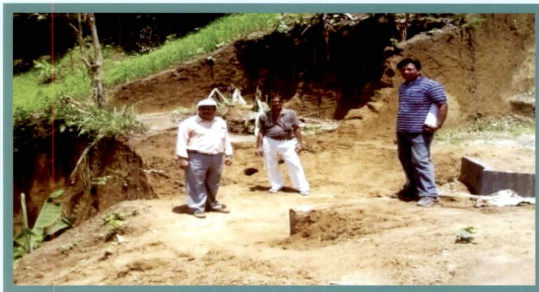
Earthen dam and spillway under construction in Saihapui MI Project under Kolasib division
