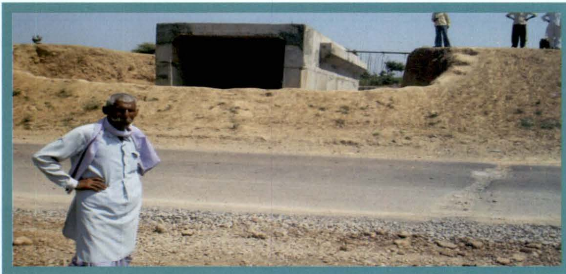
Rajghat Canal Project – Incomplete canal crossing bridges of NH-26 at Asaupur Minor
