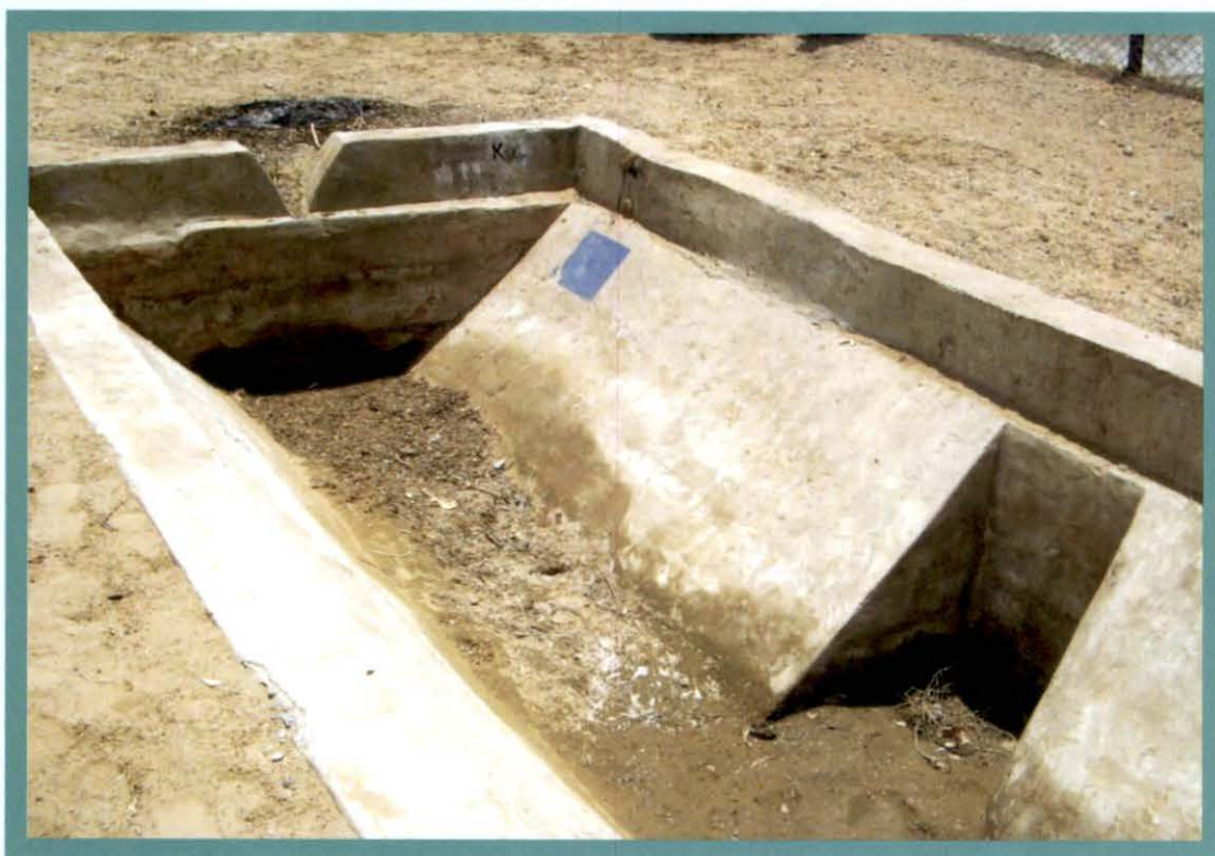
Narmada Canal Project – Incomplete work in the Inlet of Diggi No.5 Basan Minor at tail 3.701 km – Vank Distributary
