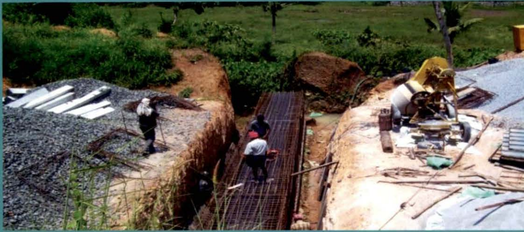
Kallada Irrigation Project - Kerala : Poovattoor Distributary- Bottleneck work in the Railway portion – Work just started
