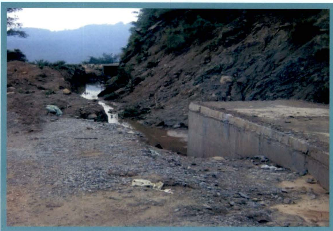
RCC box not done
