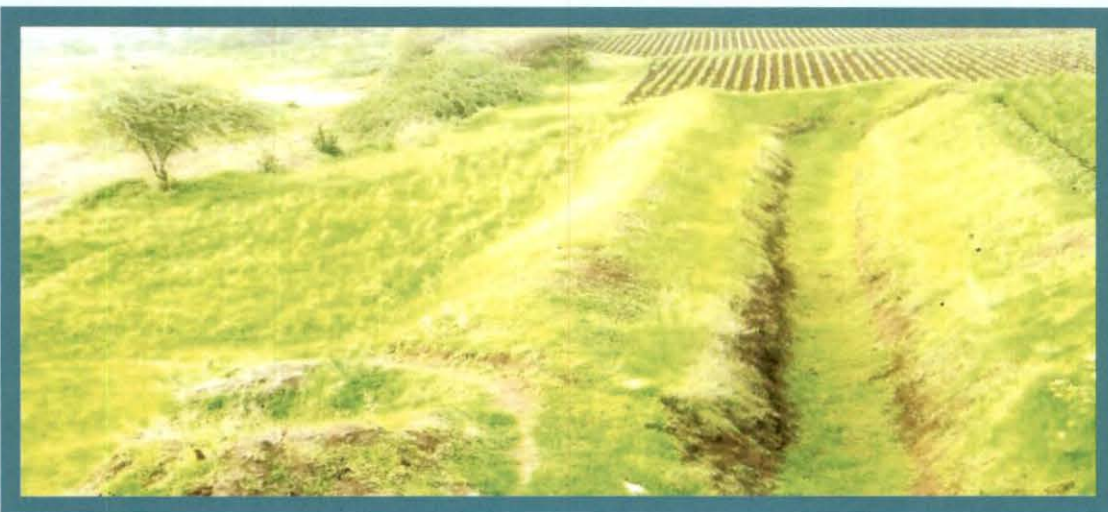
Chaupala MI Project – Canal work stopped due to land acquisition problems and obstructions from framers
