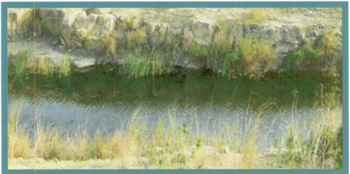
Right Bank Canal (RBC) of Rengali Irrigation Project (RIP) – Failure of slope and slippage of embankments at RD 34.24 km of RBC
