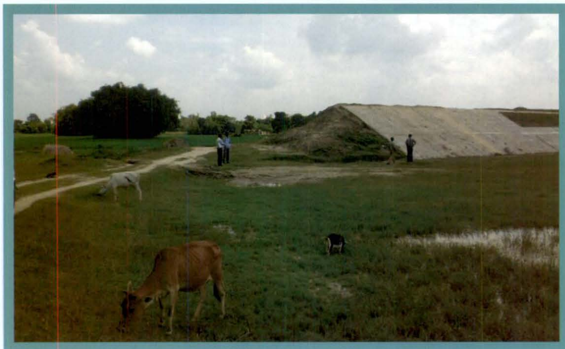
Dauk Nagar Main Canal of TBP at Ch. 63.585 where no trace of canal water was observed due to land dispute in Uttar Dinajpur District
