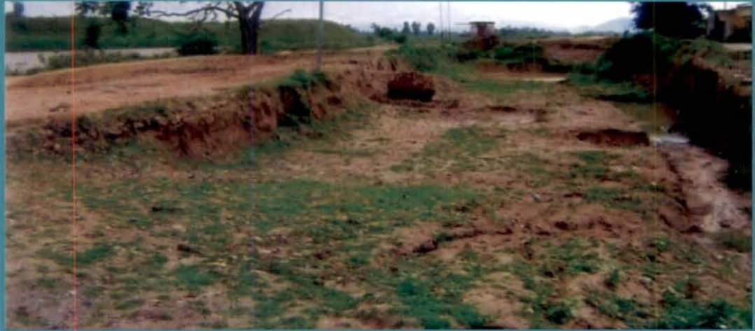
Sone Canal Modernisation Project (SCMP) – Bihar : Incomplete Western Parallel Link Canal
