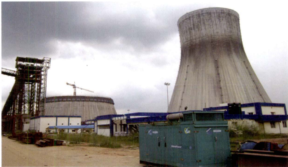
Picture 4: Incomplete NDCT-I and Complete NDCT-II at RTPS
