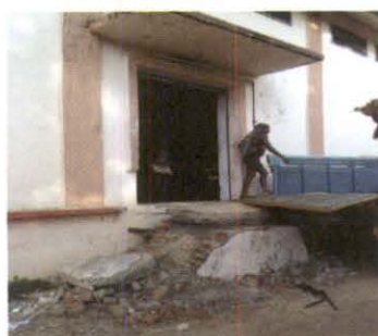
Picture 8: Damaged platform in Tiruvarur WH
