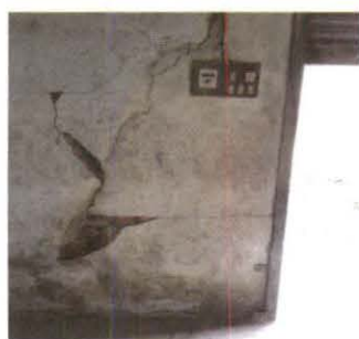
Picture 5: Cracks in wall – Salem Town WH
