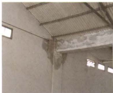
Picture 6: Leaky roof in Namakkal WH
