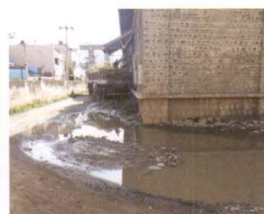
Picture 10: Damaged approach road in Vellore WH
