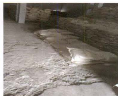
Picture 7: Damaged floor in Nagapattinam WH
